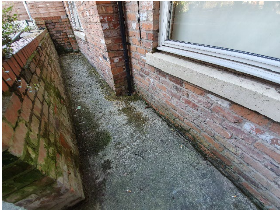
Photo 25: Moss covered concrete.
