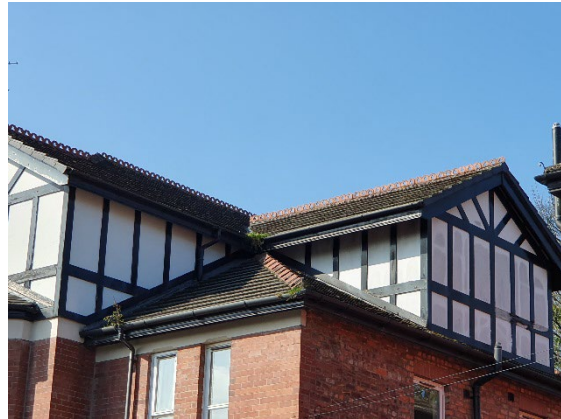
Photo 2: Mock Tudor to third floor.
