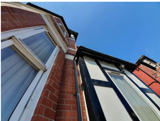
Photo 11: Gutters overflowing with debris.
