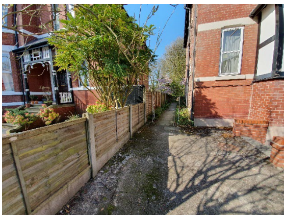
Photo 17: LHS timber panel and concrete post fence.
