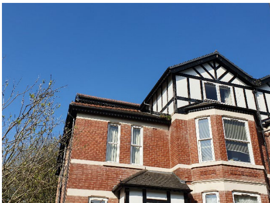
Photo 5: Mock Tudor to third floor.
