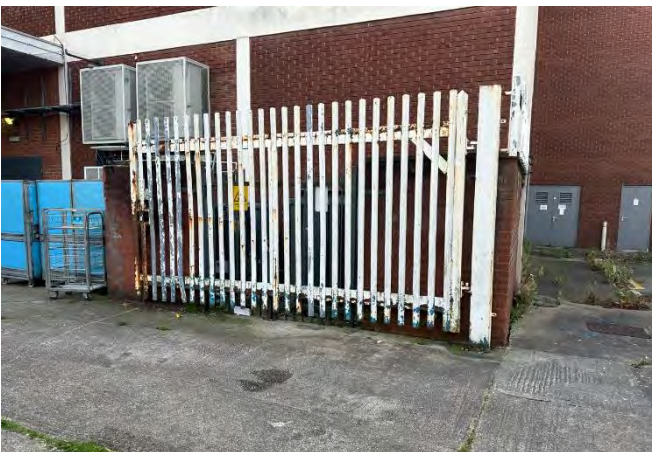
3. Electrical substation in north of site behind Graeme House.
