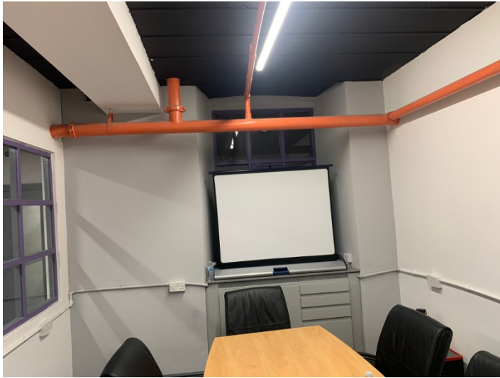
Image of existing sprinkler system pipework.
