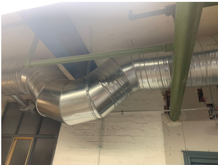
Image of existing ventilation
