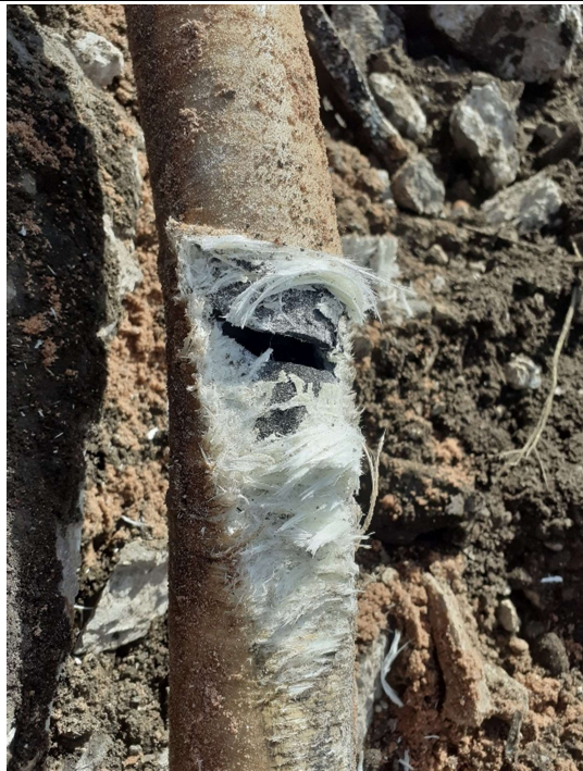
Plate 34: Monday 5 th September 2022. Asbestos lagging on pipe found on site during excavations.
