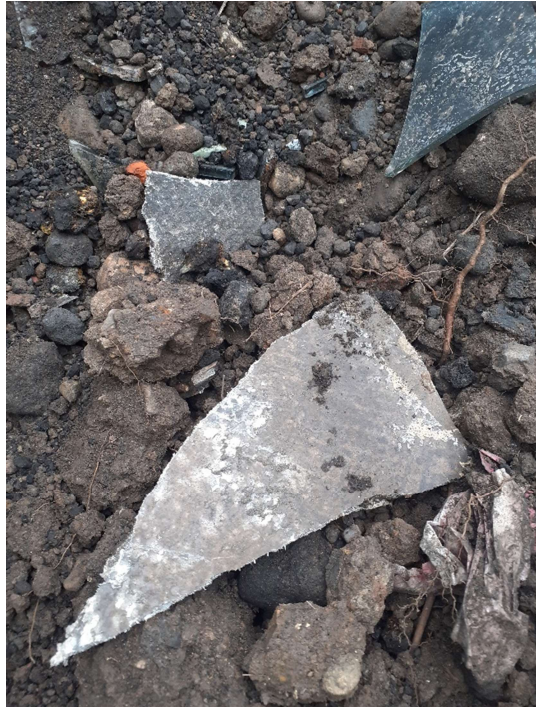
Plate 23: Friday 25 th August 2022. Asbestos fragments found in made ground excavations.
