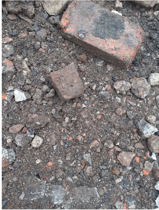
Plate 1: Friday 25 th August 2022. Asbestos hotspot 1 – image of the base.
