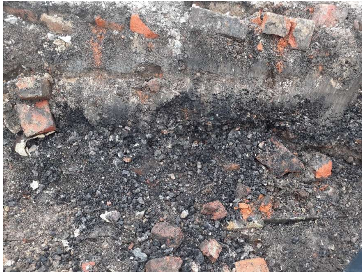
Plate 21: Friday 25 th August 2022. Asbestos hotspot 4 – image of the western side.
