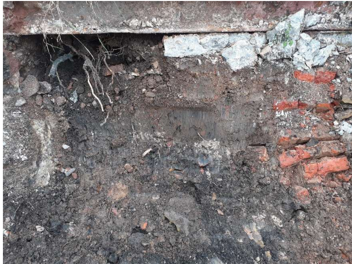
Plate 15: Friday 25 th August 2022. Asbestos hotspot 3 – image of the southern side.
