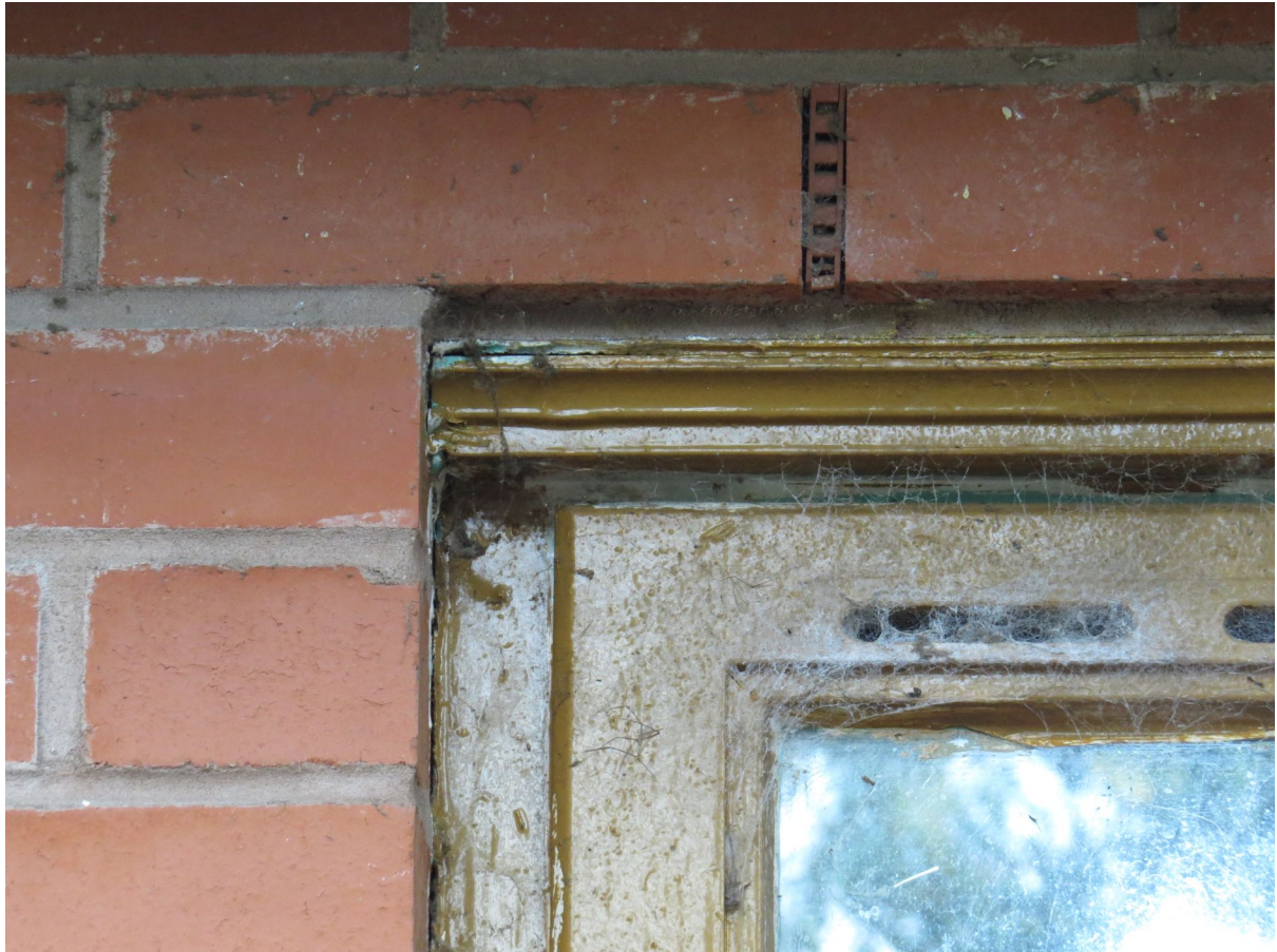
11 – Window and door frames are tightly fixed into brickwork with no viable gaps.
