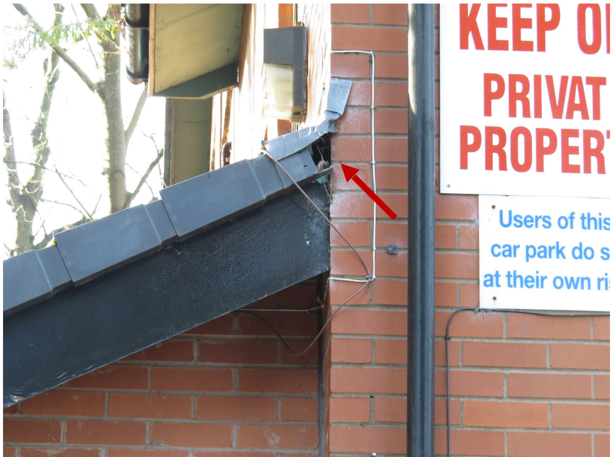
5 – Lead flashing and dry verge covers are damaged and could give access to roosting bats.
