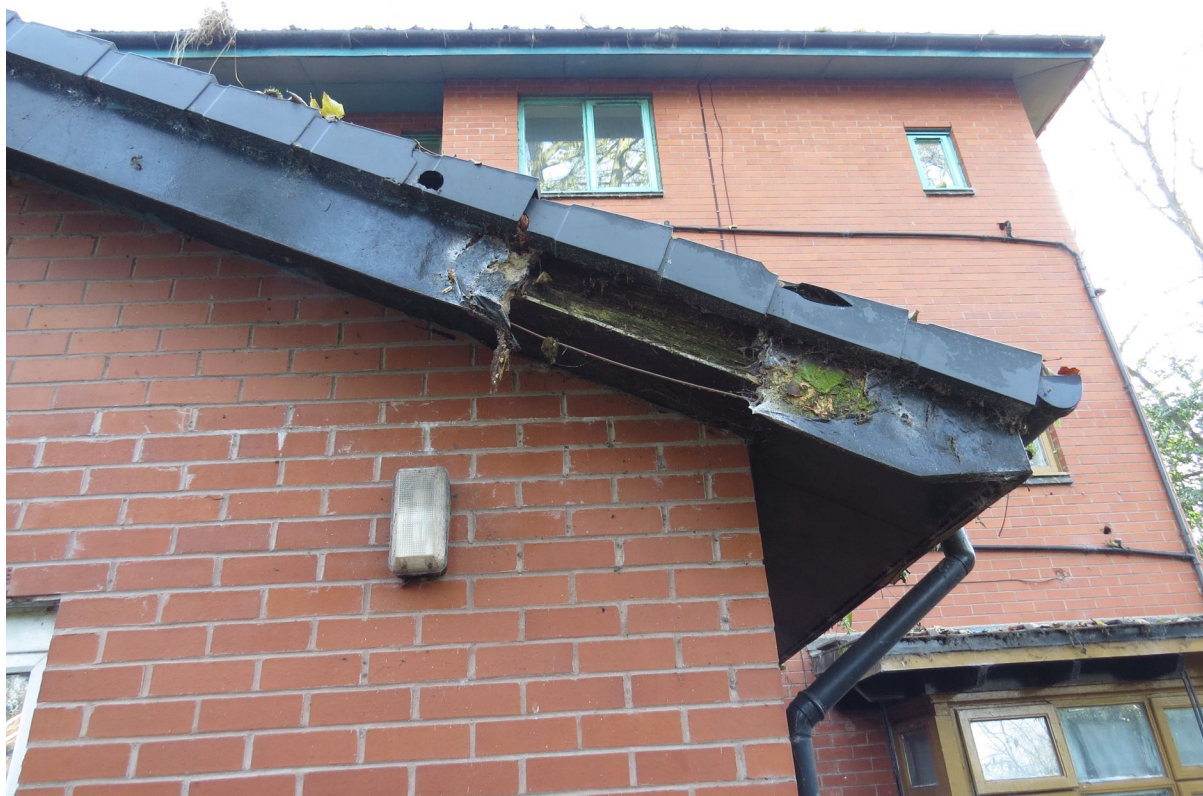
3 – Damaged fascia boards and soffits.
