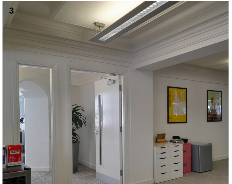
Plaster cornice in office area
