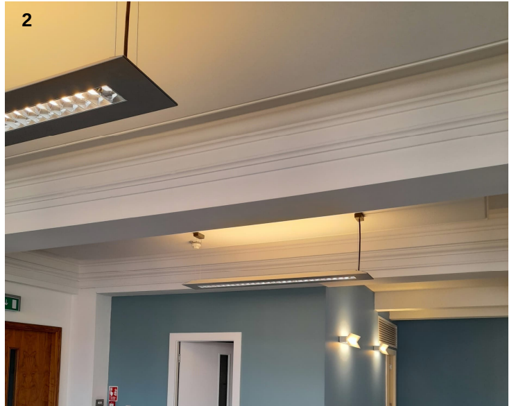
Plaster cornice in office area
