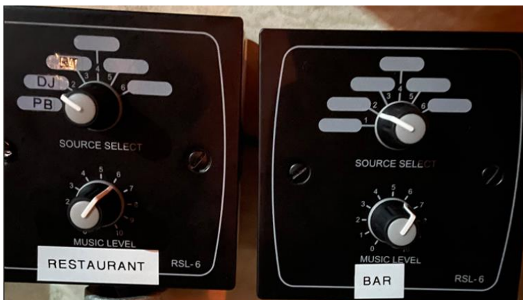
Figure 3 Installed RSL-6 type controllers (restaurant and bar spaces)
