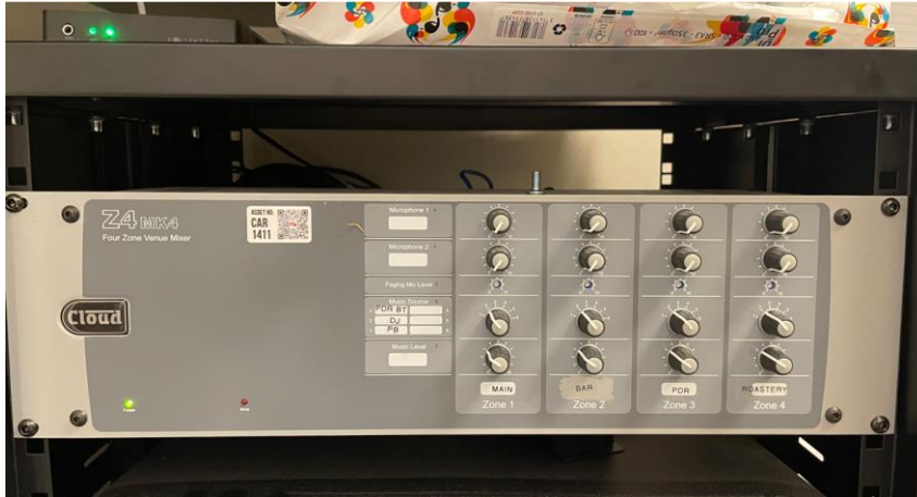
Figure 2 Installed Cloud Z4MK4 four zone volume control unit
