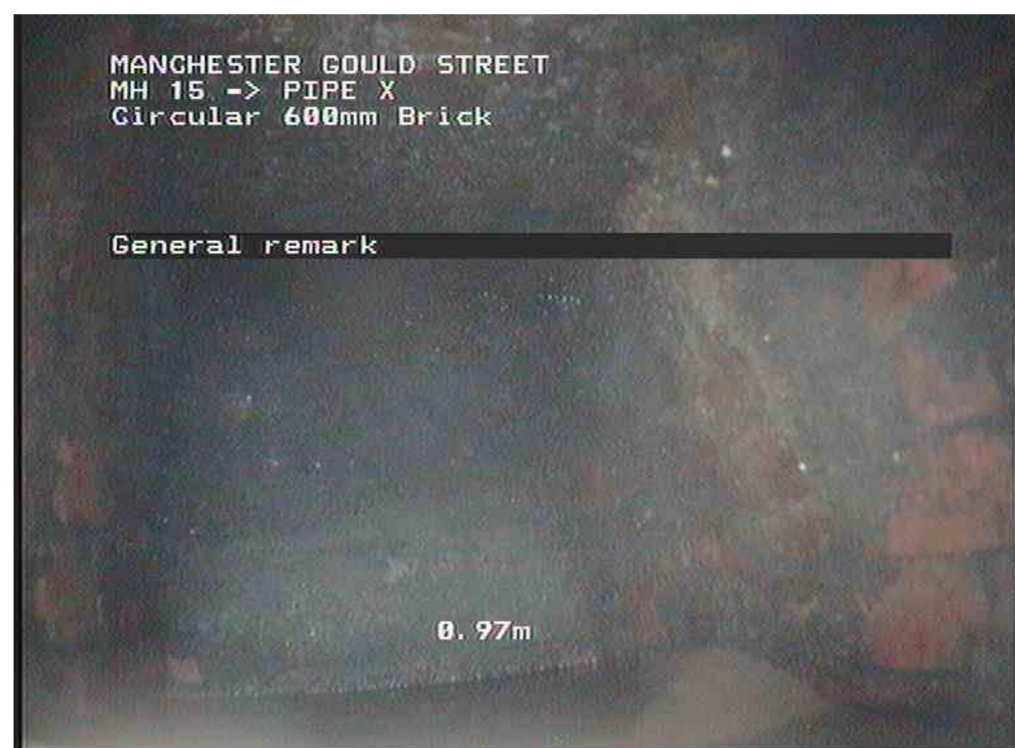
MANHOLE 15 CONDITION AT INVERT LEVEL, NO PIPE VISIBLE, SURVEY TERMINATED
