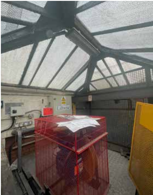
Motor Room – Image 1
