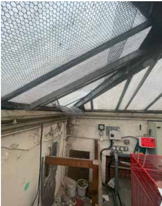
Motor Room – Image 3
