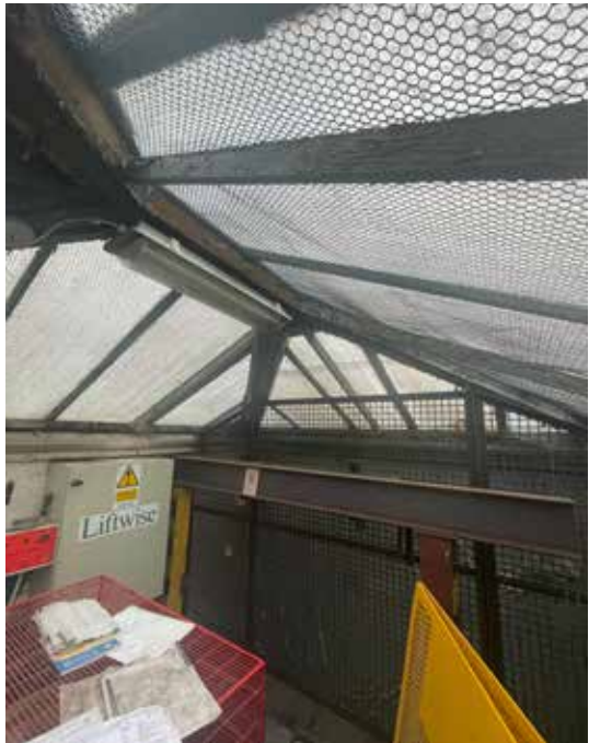
Motor Room – Image 2
