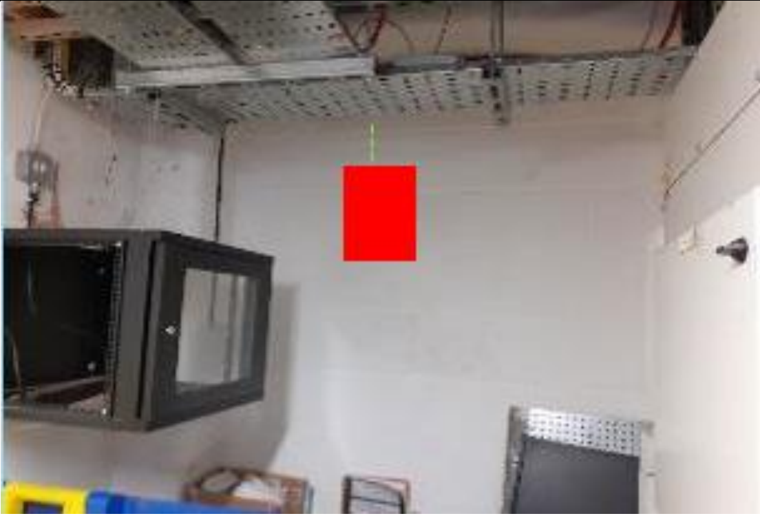
Photo 5: New cable box in bin store
