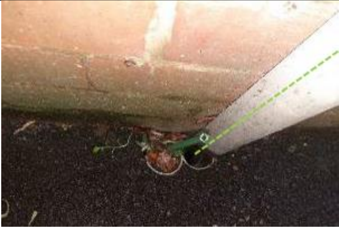
Photo 3: Cable travelling up the wall using existing duct protected by galvanized capping
