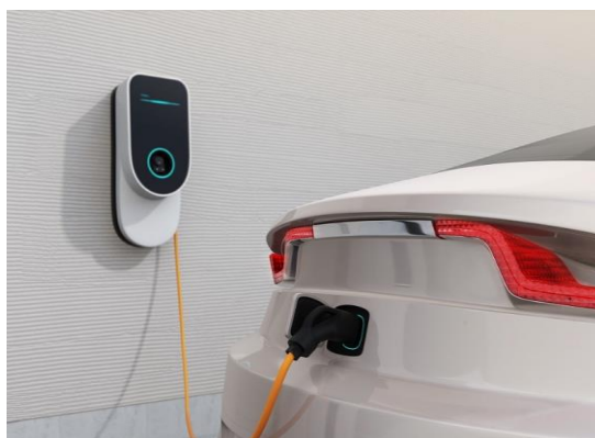
Figure 8 - Example of EV Charging
