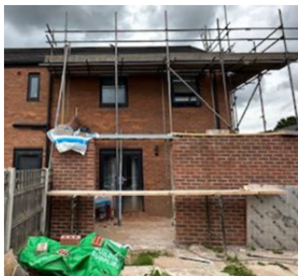
Figure.2 Unauthorised works (photo dated July 2024)
