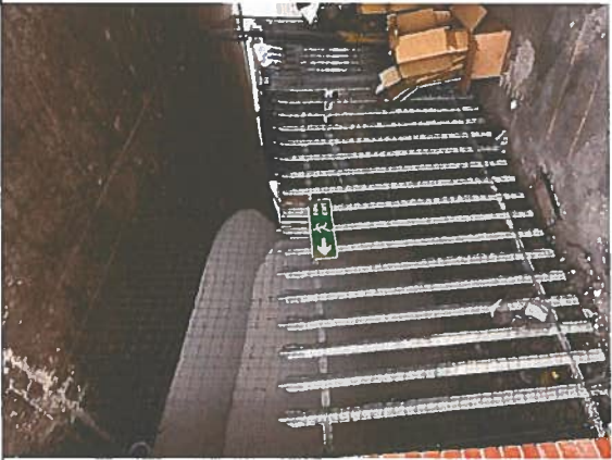
Underside of access ramp – note potential risk of vermin
