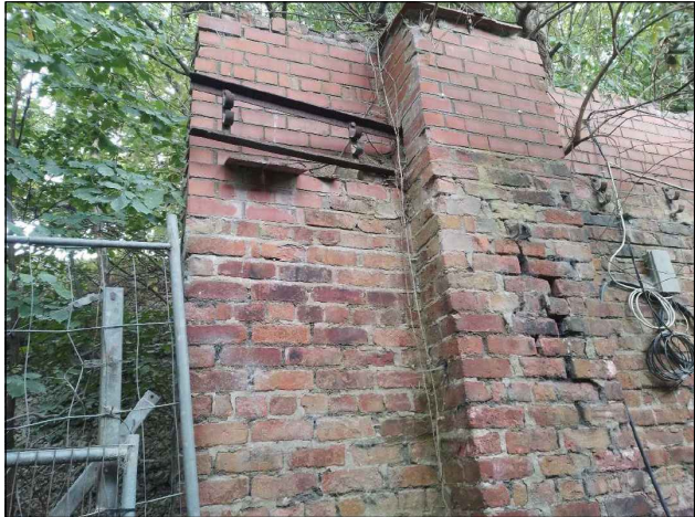
U2 - No brick work to left of image, fence to be replaced as Hydrock recommendation.
