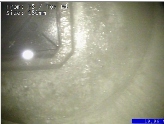
Finish node type, manhole, reference F4
