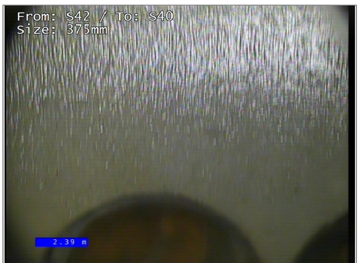
Connection other than junction at 11 o'clock, diameter 150mm
