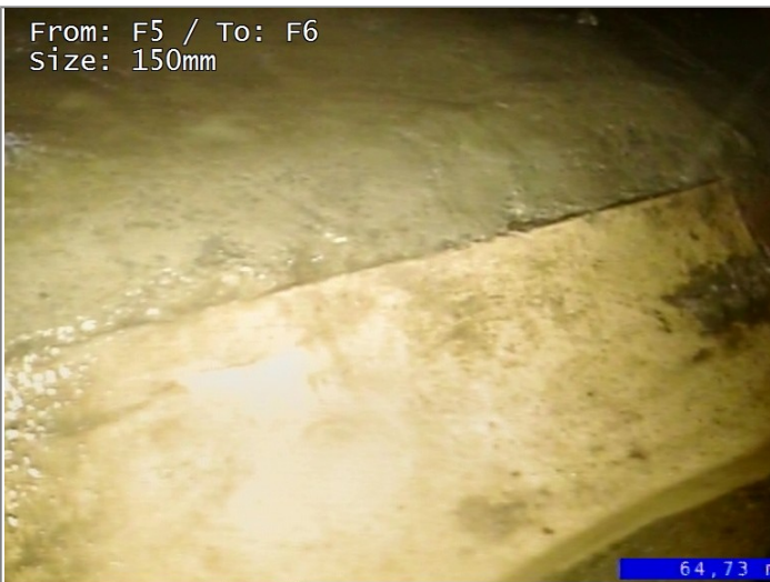
Finish node type, manhole, reference F6
