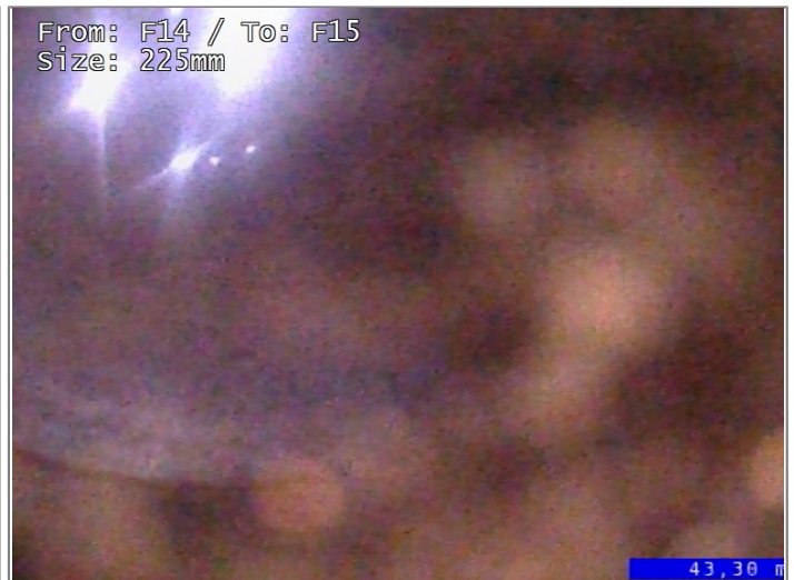
Finish node type, manhole, reference F15
