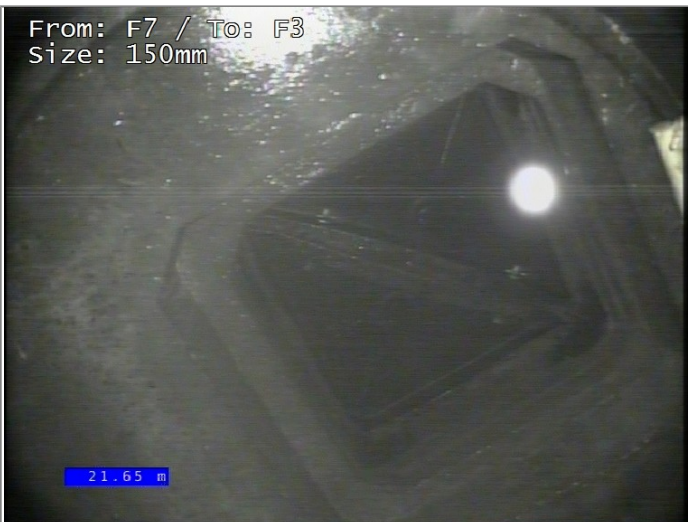
Finish node type, manhole, reference F3
