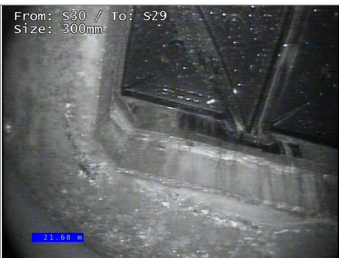
Finish node type, manhole, reference S29
