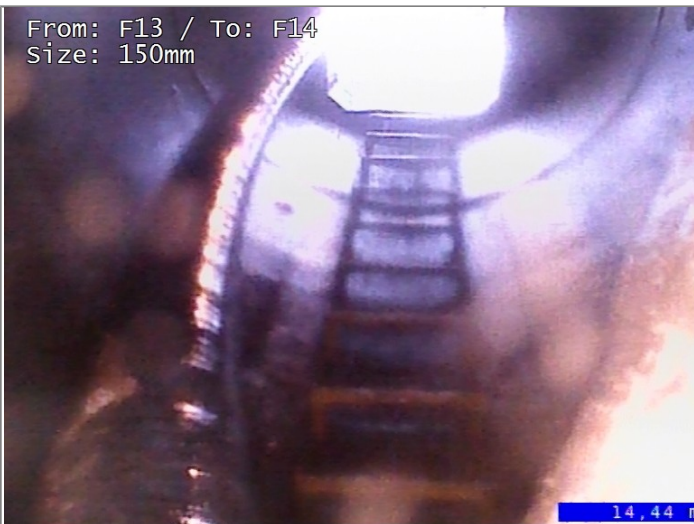
Finish node type, manhole, reference F14
