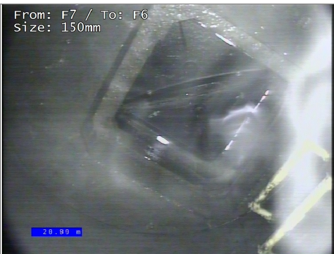
Finish node type, manhole, reference F6
