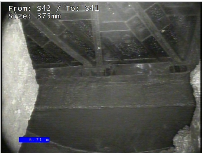
Finish node type, manhole, reference S41
