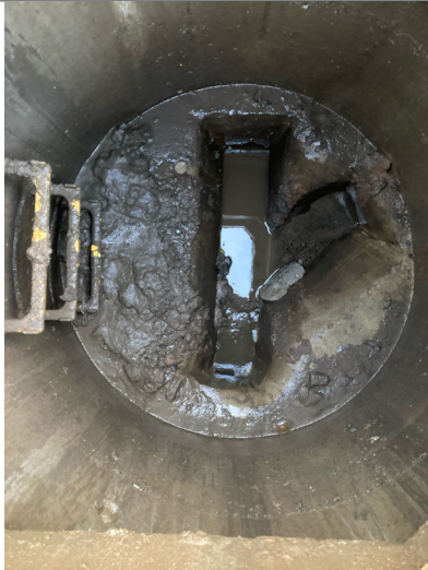
Other Site Photos: Grout in foul line
