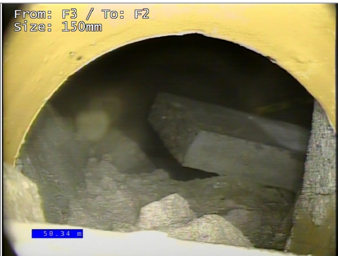
Finish node type, manhole, reference F2
