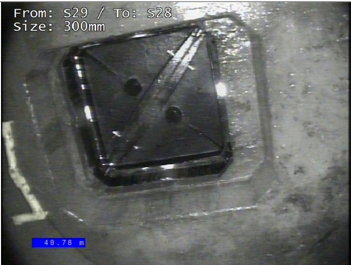
Finish node type, manhole, reference S28
