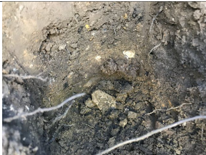
Photograph 8: View of soil in capping layer excavation in rear garden of Plot 23. No membrane is present, and topsoil has been laid straight onto made ground.
