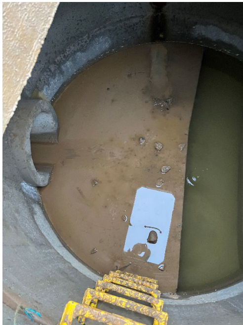
View of incoming pipe into Hydro-Brake MH
