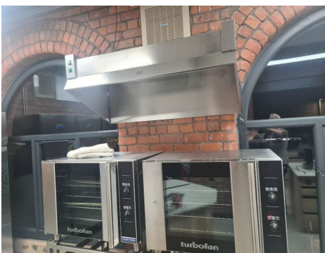
Lincat electric fume filtration canopy above the two convection ovens
