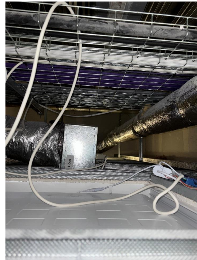
Photograph 9: B1 loft/crawl space occupied by cables and piping.
