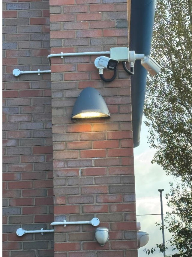
Photograph 11: view of the outdoor lighting which is consistent throughout the site.
