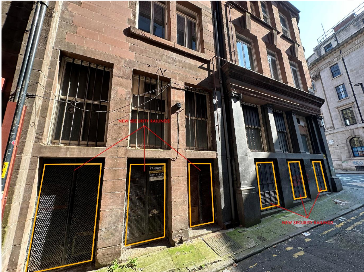
Photo showing Four Yards windows with security railing additions.
