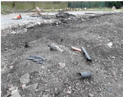
Item 13 - Trial pit 13 - Bitumen pipe buried beneath soil and associated debris to the ground
