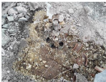
Item 17 - Trial pit 16 - Bitumen pipe buried beneath soil and associated debris to the ground
