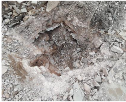
Item 20 - Trial pit 17 - Bitumen pipe buried beneath soil and concrete slab
