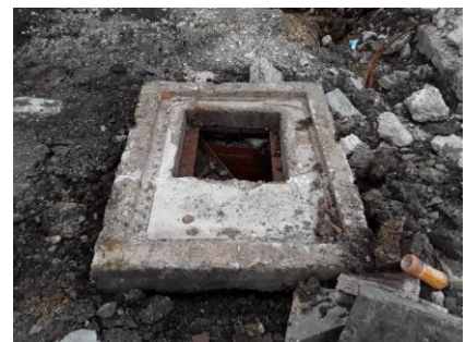
Item 18 - Foul drain, north corner - Cement used as shuttering to the underside of the foul drain entrance
