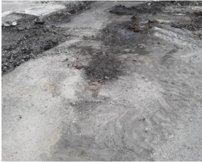
Item 19 - Area adjacent trial pit 16 - Bitumen debris to the ground
