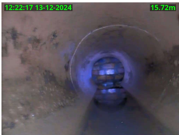
MH 14X_c5cfbed8-13d6-4d19-9def-e65f87fa8e1d_20241213_132 838_904.jpg, 00:01:21, 0.00 m Crack, circumferential from 7 o'clock to 5 o'clock
