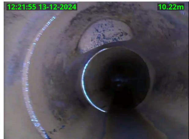
MH 14X_96301134-c358-4c4a-b97f-c43d5f708b58_20241213_13 2617_984.jpg, 00:00:59, 0.00 m Junction at 11 o'clock, 150mm dia
