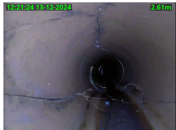
MH 14X_b49e79ca-91c7-4a55-a4d0-64c3836b8e3e_20241213_1 32359_309.jpg, 00:00:29, 2.61 m Fractures, multiple from 12 o'clock to 12 o'clock
