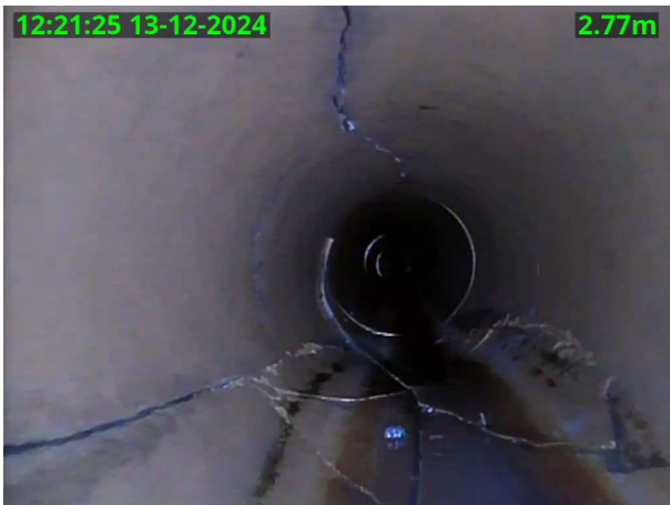
MH 14X_625bcc0b-507e-4196-946c-ad69b5581467_20241213_1 32410_047.jpg, 00:00:29, 2.77 m Deformed sewer or drain, 5%
