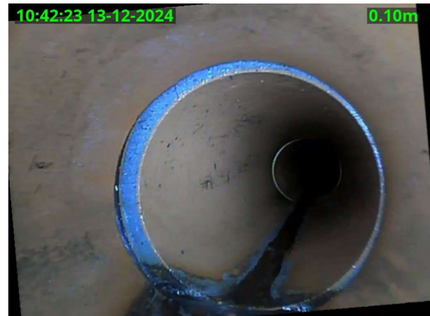
MH 25X_f5a04bc5-c807-455a-9cfc-f273a1b82d66_20241213_131 736_616.jpg, 00:00:12, 0.10 m Joint displaced, medium
