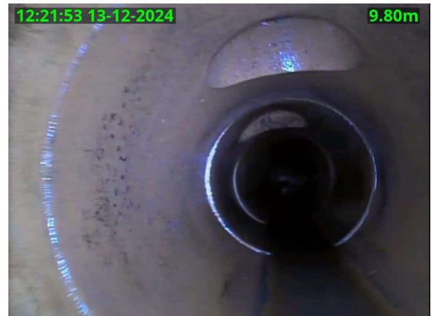
MH 14X_b6d000e5-2370-4220-87f3-02461de9b09d_20241213_1 32520_770.jpg, 00:00:57, 9.80 m Junction at 12 o'clock, 150mm dia
