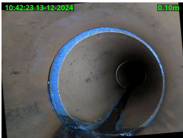
MH 25X_c25be6f0-a5b6-48f4-ac28-247a3d333981_20241213_13 1802_748.jpg, 00:00:12, 0.10 m Line deviates right
