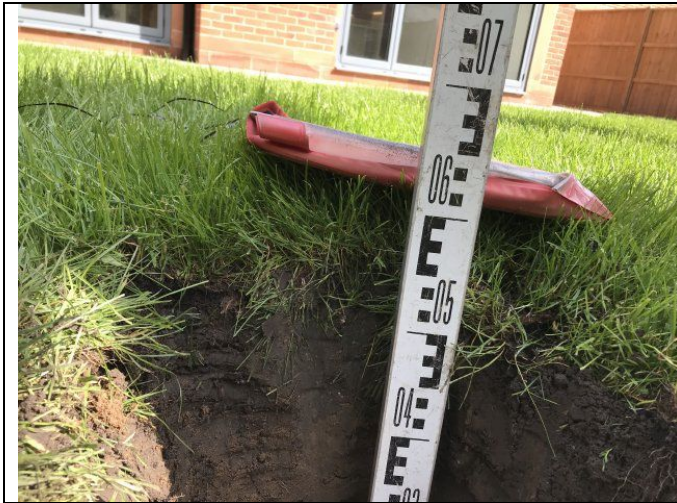
Photograph 4: Depth measurement in rear garden of Plot 19.
