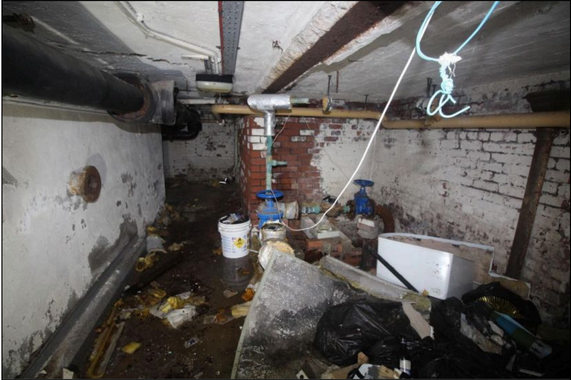
Plate 62: General view of the basement area, detailing the modern pipework that had replaced earlier cast-iron pipework
