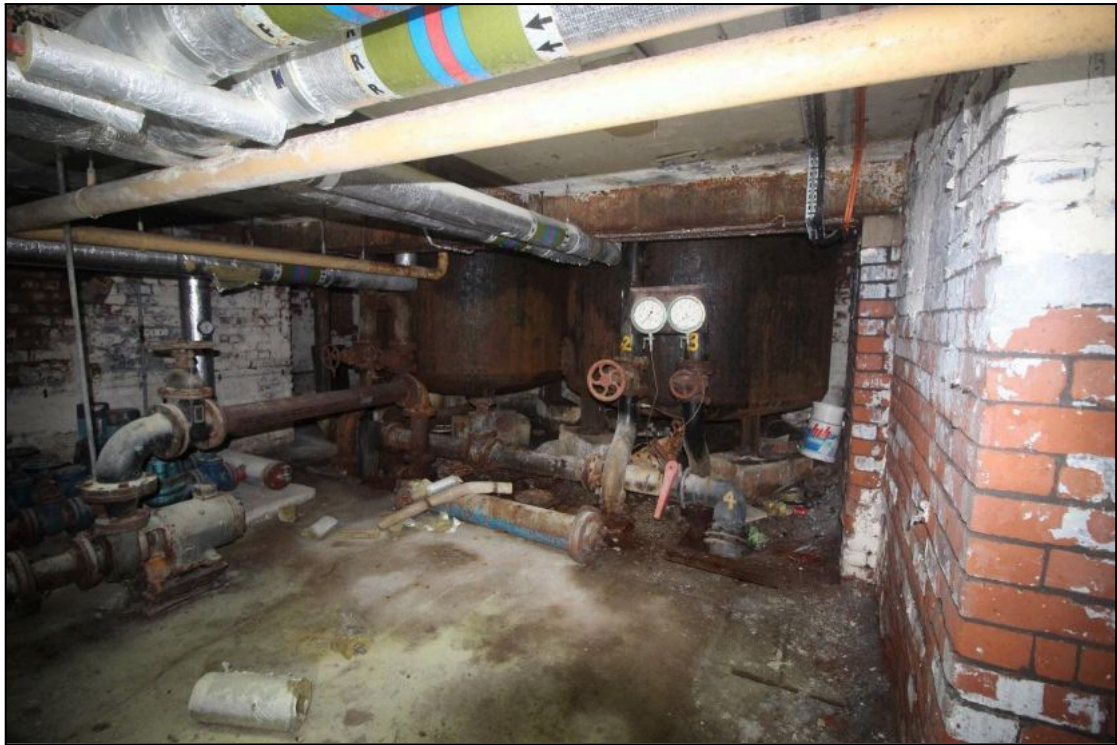
Plate 63: The two calorifier tanks within the basement
