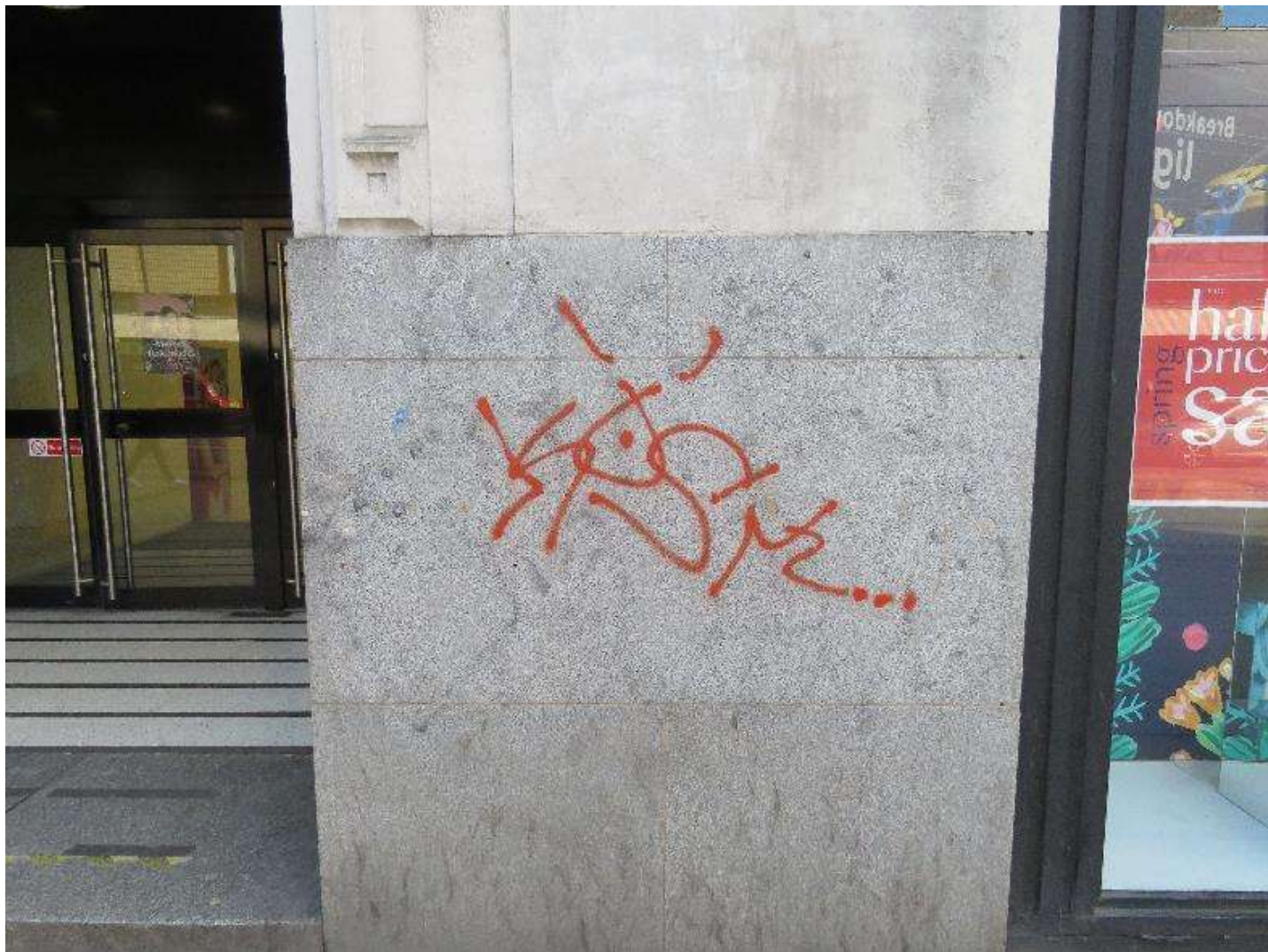
Fig. 6: View of the granite cladding to the entrance on High Street, with graffiti and soiling.
