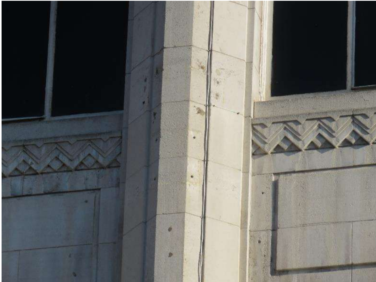
Fig. 8: Redundant fixings will need to be removed and the holes filled with a lime-based mortar repair, unlike the previous cement based repairs that have been undertaken.
