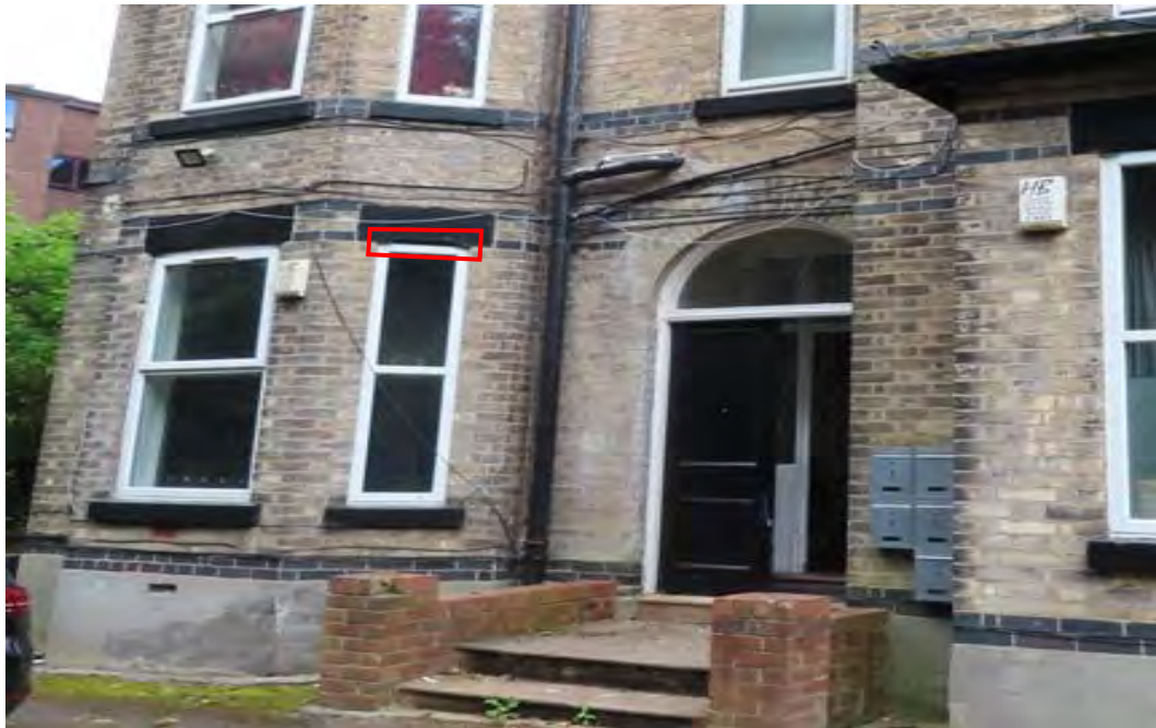
Photograph 3 – PRFs present between concrete lintel and window frame at Building 1.
