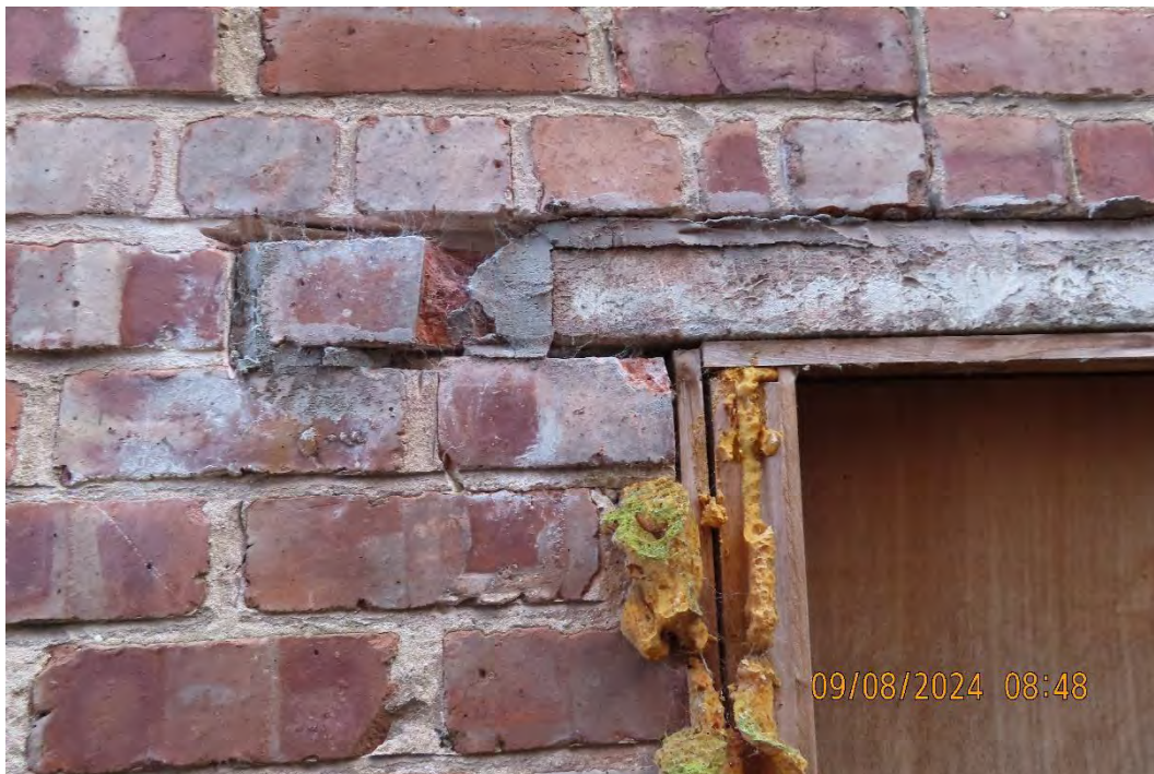
Photograph 15 – Cobwebbed gaps at the concrete lintels of the garage of Building 3.
