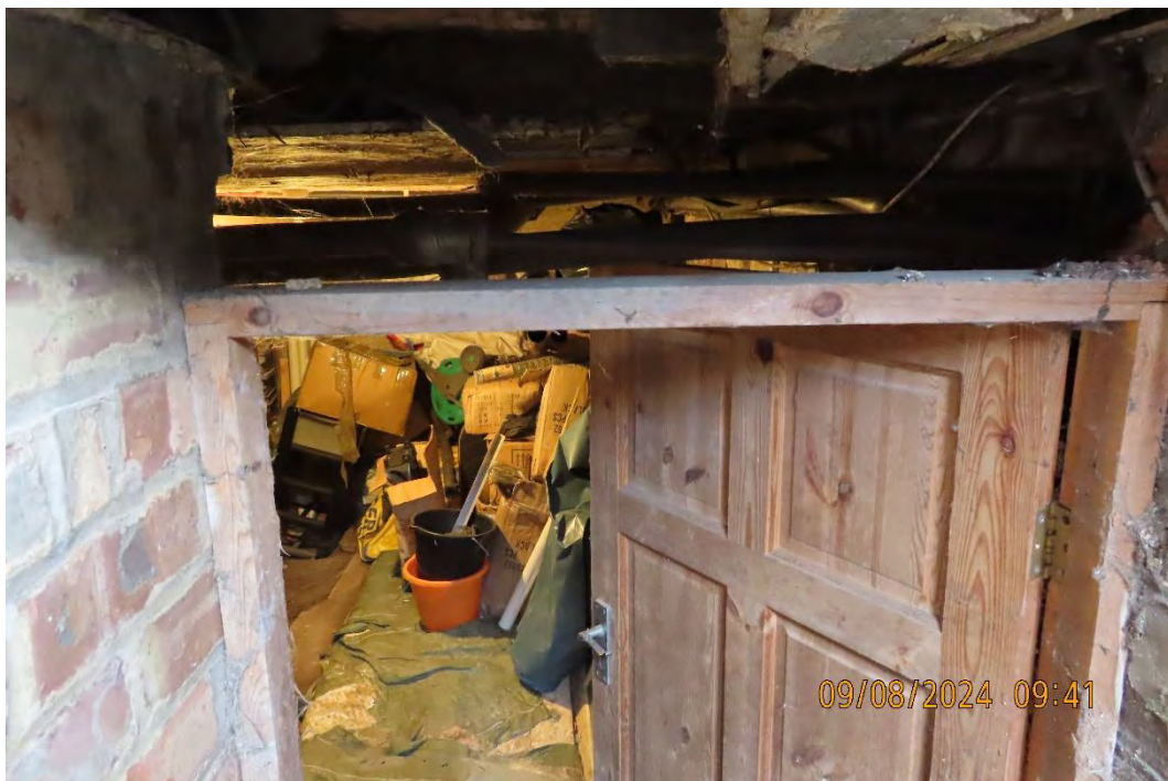
Photograph 20 – Large gap above the timber doorframe that could be utilized as an access point.
