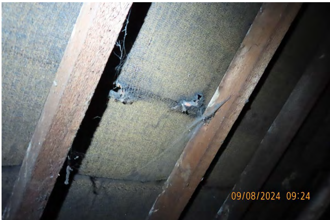
Photograph 22 – Bitumen lining featuring several tears.
