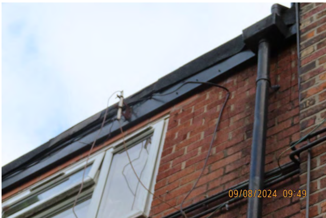
Photograph 4 – Gaps present underneath the lifted sections of bitumen roof felt at Building 1. Roost 2 is present under the raised roof felt.
