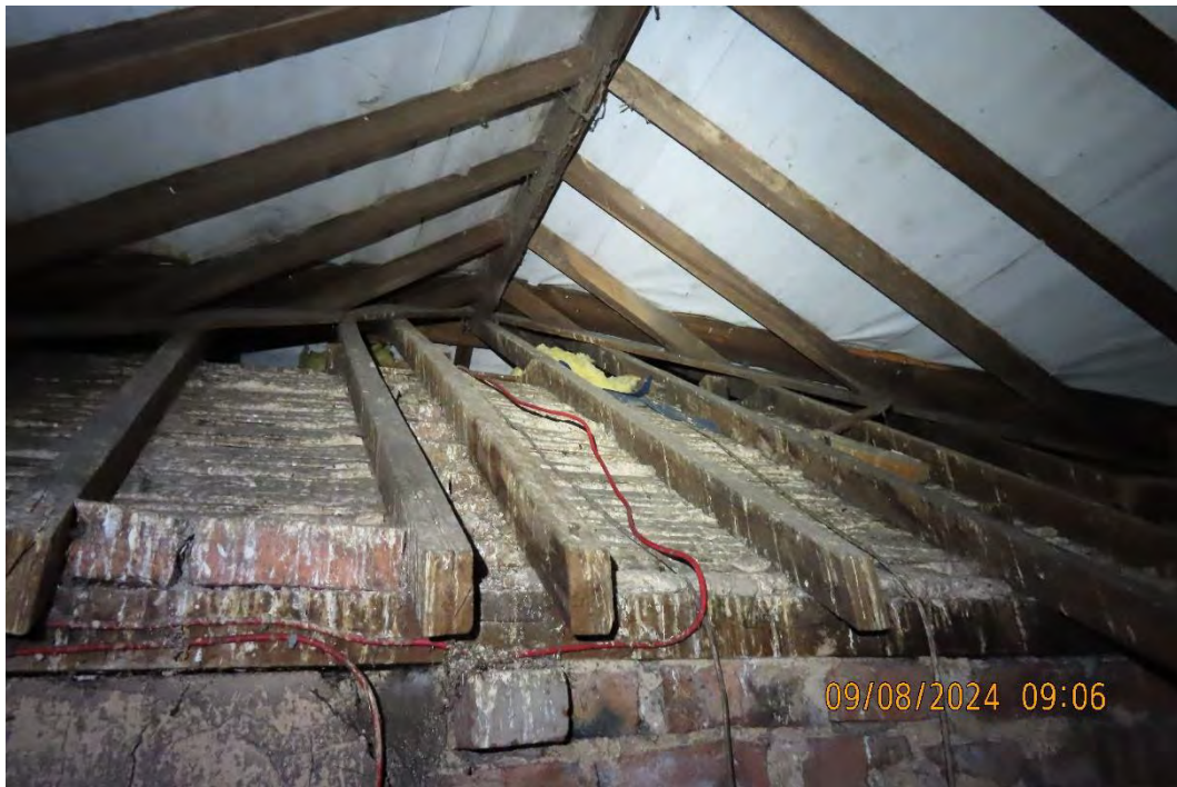
Photograph 18 – Breathable roof membrane in good condition with no visible tears. Also present are large concentrations of pigeon excrement.
