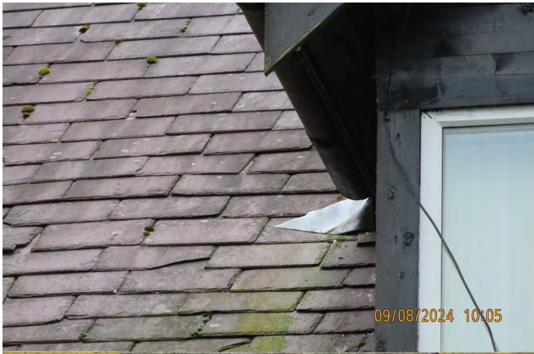
Photograph 12 – Lifted lead flashing creating a suitable gap for roosting bats at Building 3.
