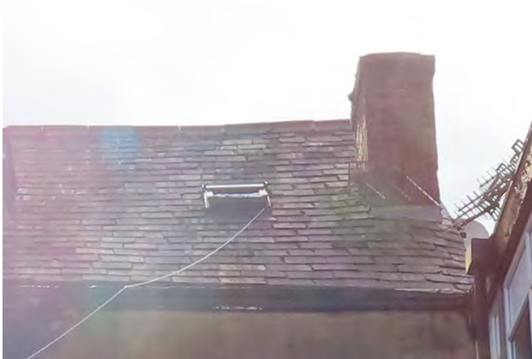
Photograph 8 – Uneven and lifted roof tiles of Building 2. Most notably towards the gable end and around the chimney of Building 2.
