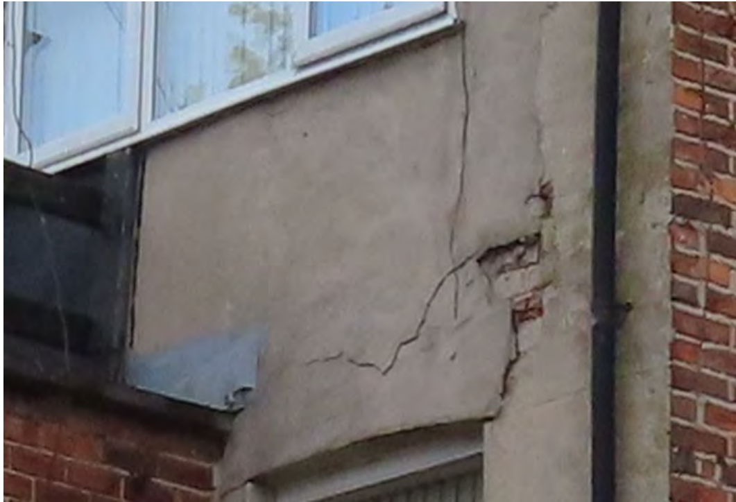
Photograph 13 – Section of mortar cladding with gaps and crevices present at Building 3.
