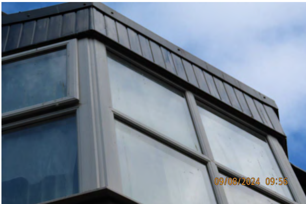
Photograph 10 – Gaps present underneath the overhanging metal lining at Building 2.
