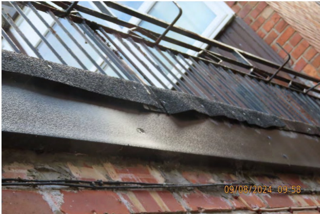
Photograph 9 – Numerous sections of lifted bitumen roof lining at Building 2.
