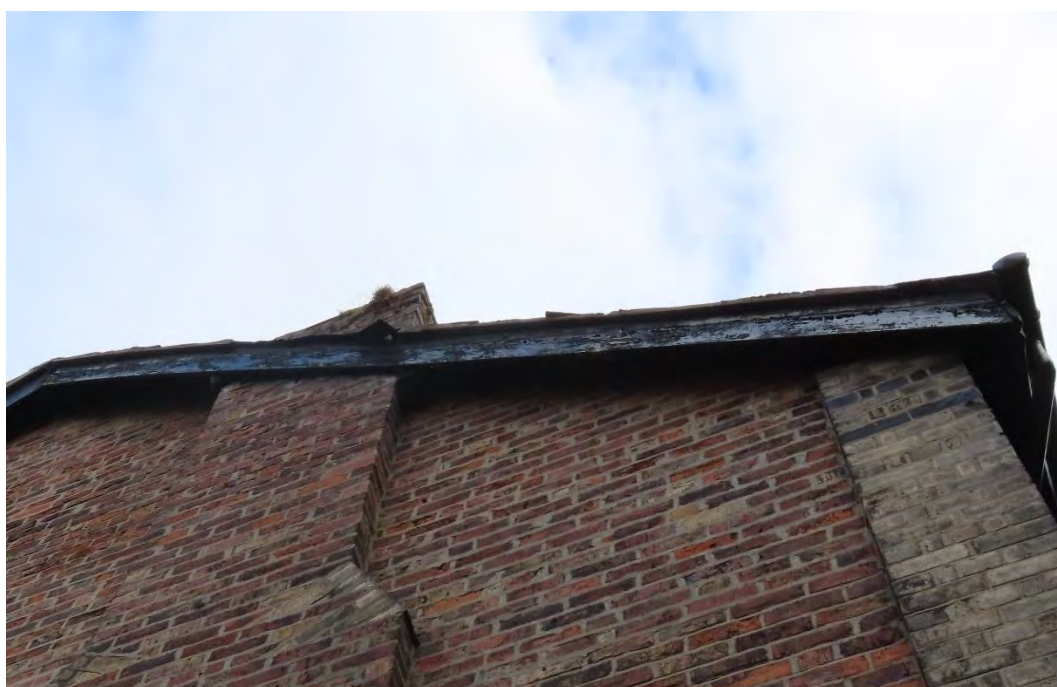
Photograph 2 – Displaced roof tiles at the south-western gable end of Building 1.
