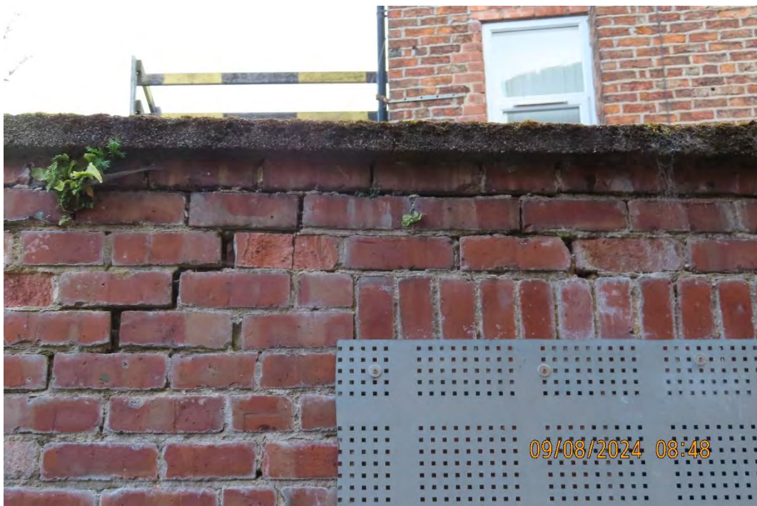
Photograph 14 – Gaps present within the brickwork and mortar at Building 3.
