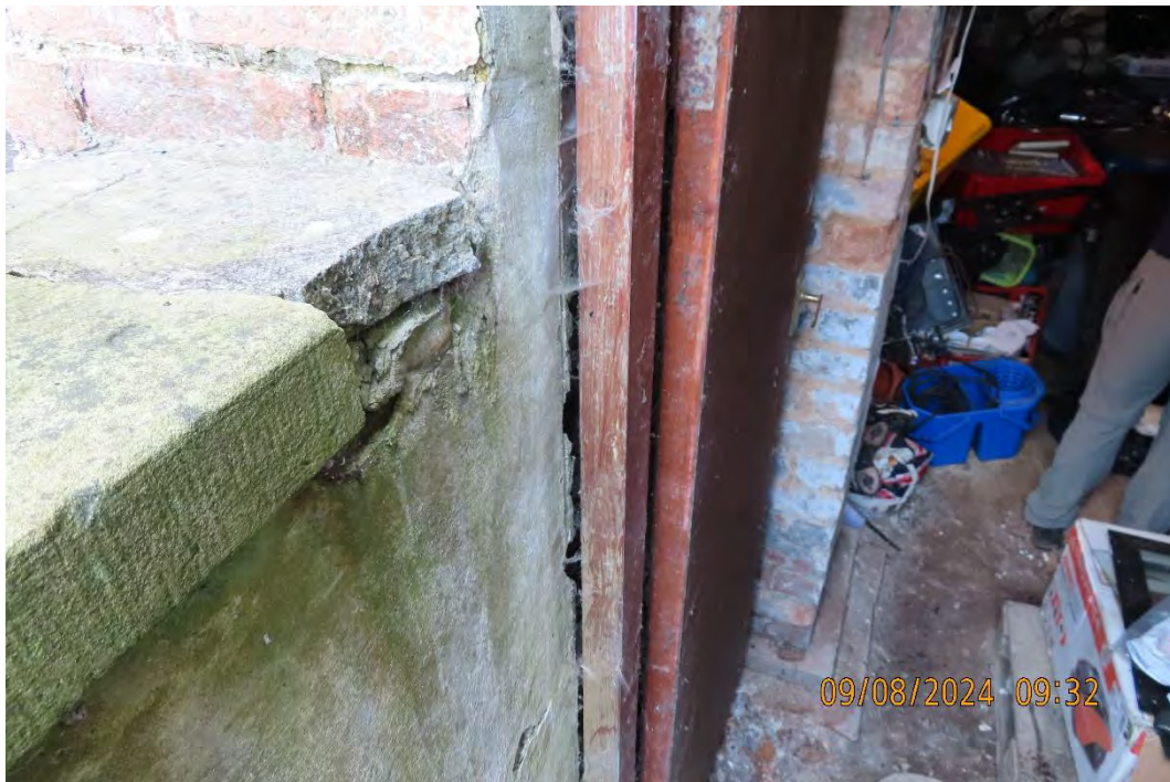
Photograph 24 – Gaps present between the timber doorframe and brickwork.
