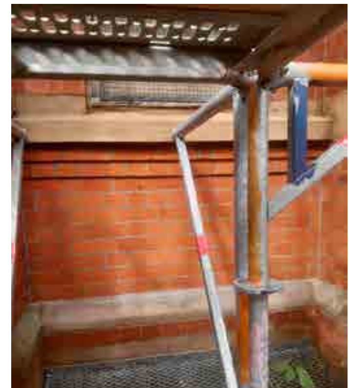
images illustrates the 'after' condition
