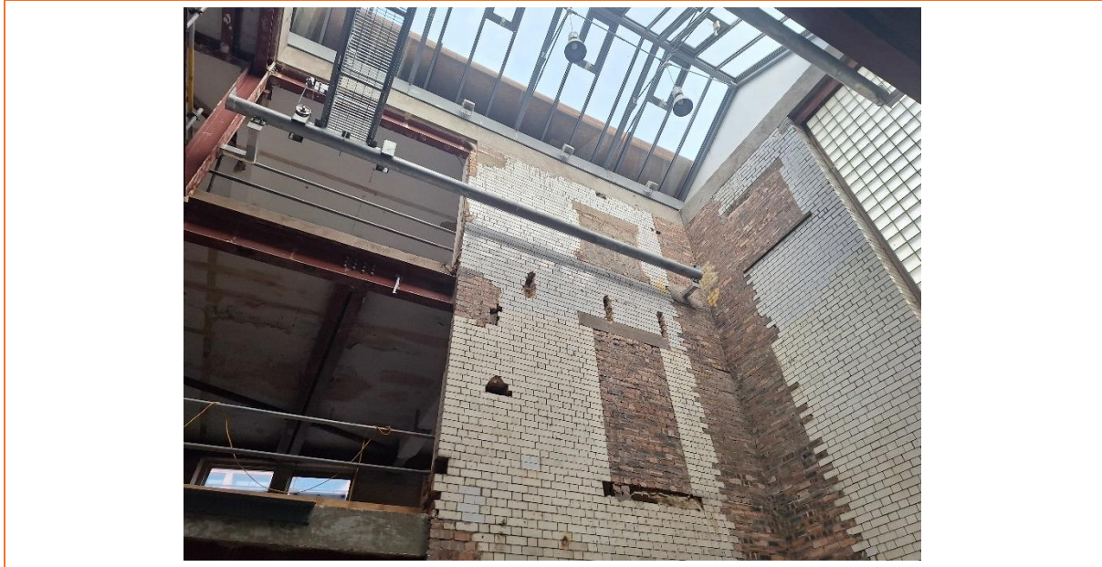
Figure 14 Showing Internal Damaged Brickwork
