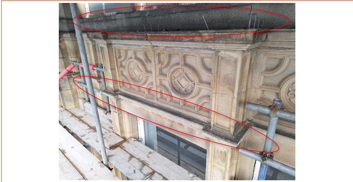
Figure 17 Showing Bird Deterrent Wire and Spikes
