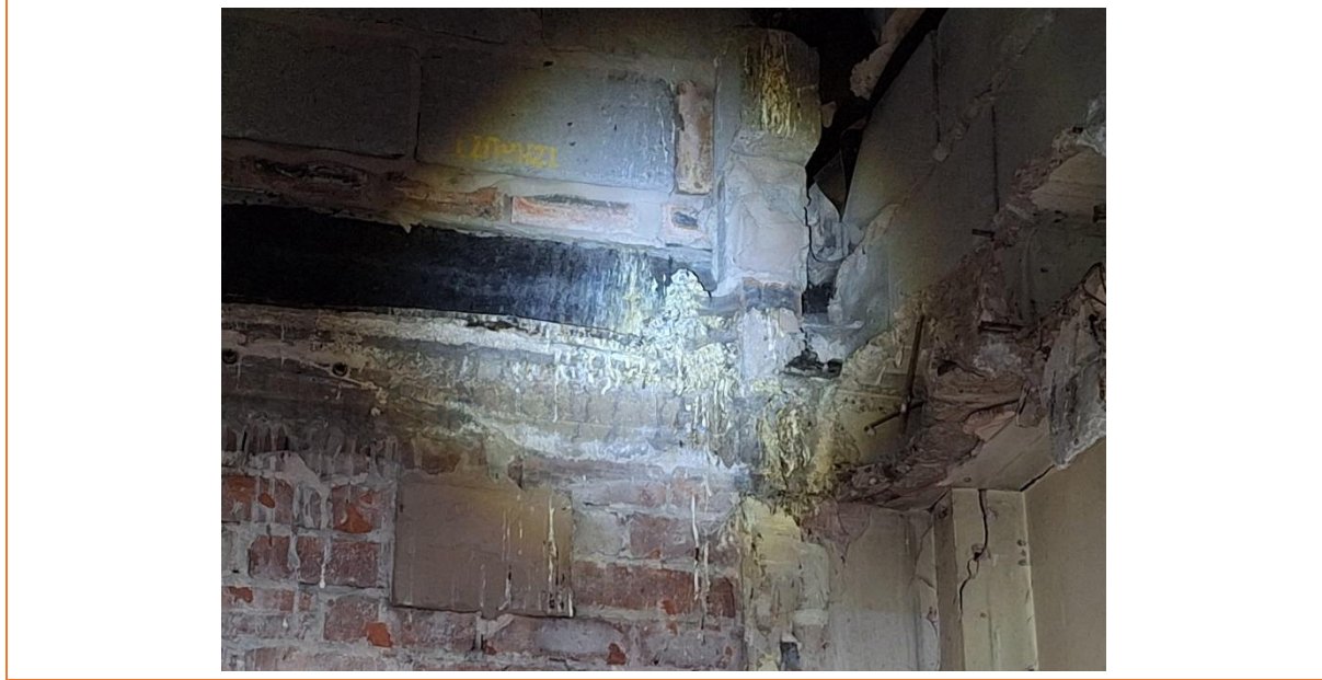
Figure 15 Showing Bird Droppings
