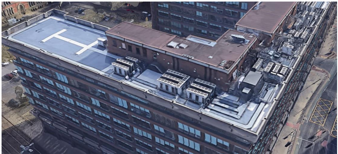
Typical Location of existing Mechanical Plant – Aytoun Street Elevation
