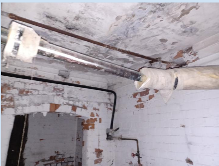
Insulation residues to wall, pipework and pipe brackets in location B1-032
