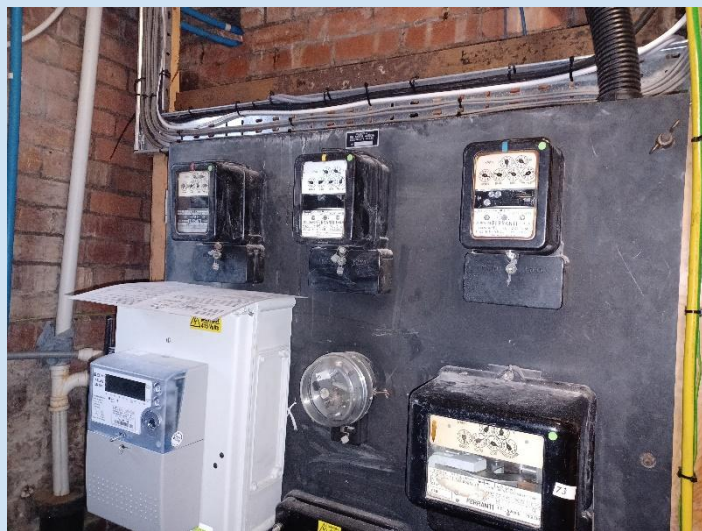
-1/B01/B1-003-electrics – Panel to electrics to be removed
