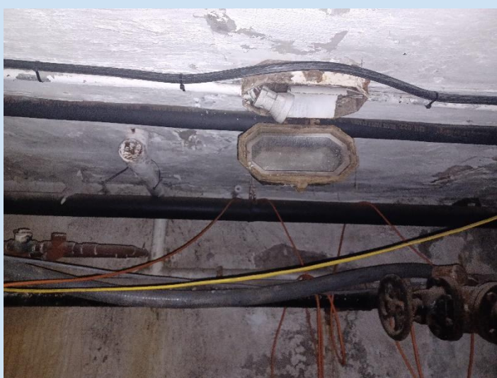
-1/B01/B1-006 and -1/B01/B1-037- basement of males 1st class swimming pool - light to be removed due to mastic
