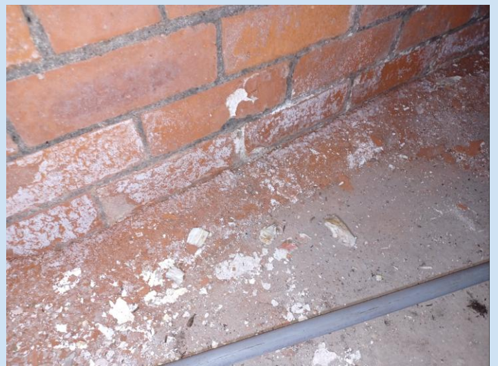
Insulation debris to the floor in location B1-035
