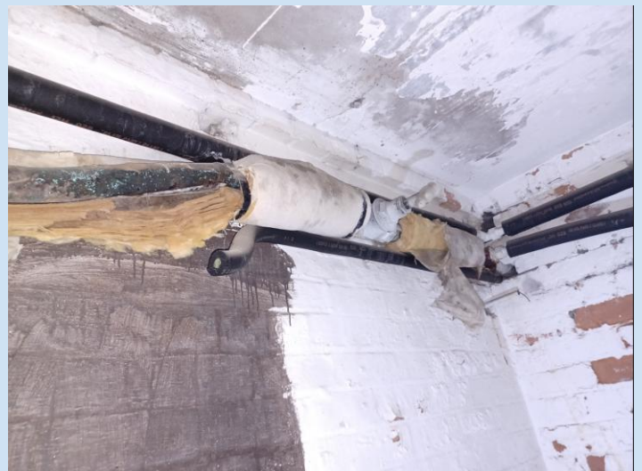
Insulation residues to wall, pipework and pipe brackets in location B1-031
