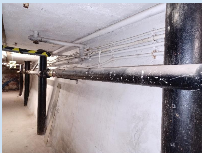
-1/B01/B1-037- basement of males 1st class swimming Pool – Asbestos cement pipe to be removed
