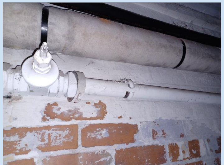
Insulation residues to wall, pipework and pipe brackets in location B1-033
