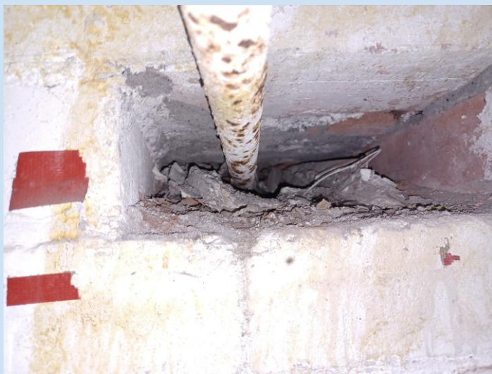
Insulation residues within pipe penetrations in location B1-035
