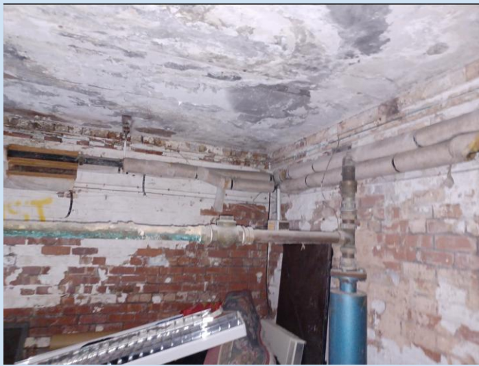
Insulation residues to pipework and pipe brackets in location B1-034
