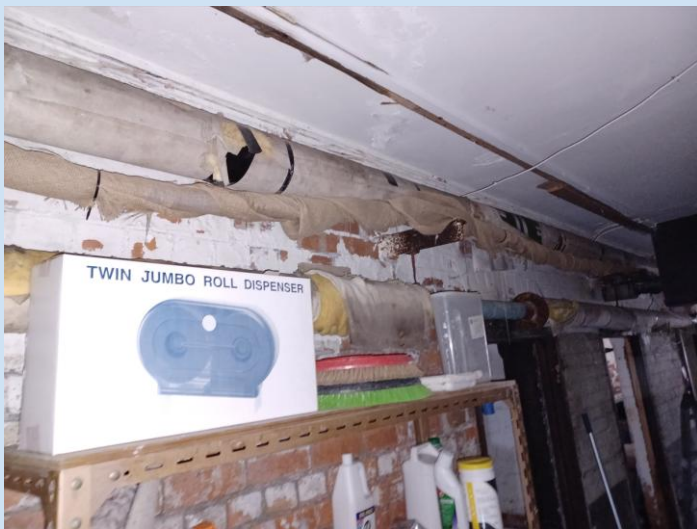
Insulation residues to wall, pipework and pipe brackets in location B1-030
