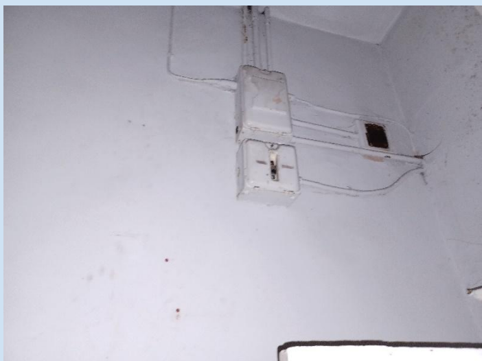
1/B01/01-012 Electrics to be removed
