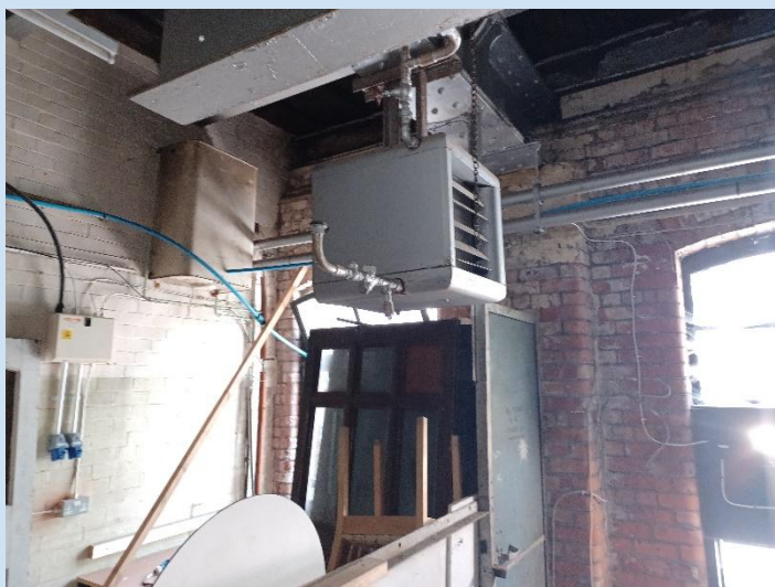
0/B02/GF-005-Electrician store - Heater to be removed
