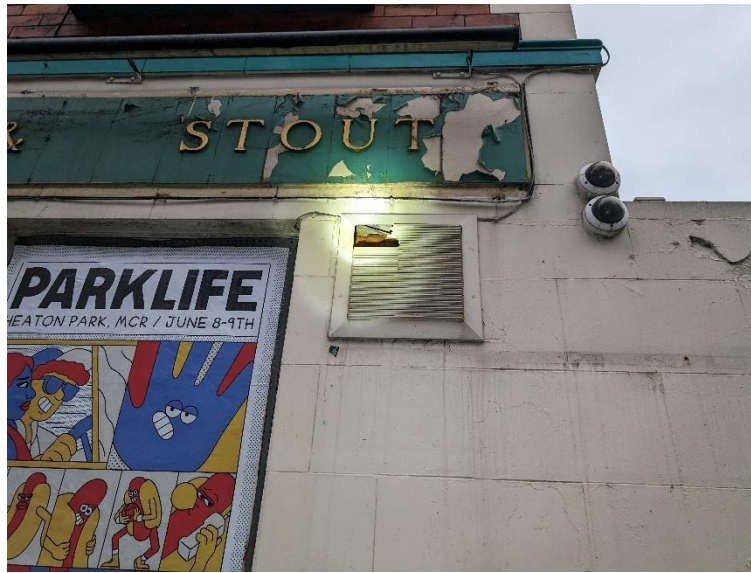
PLATE 8 SHOWING BROKEN VENT
