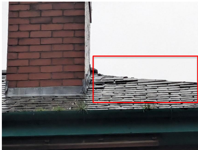
PLATE 9 SHOWING DAMAGED AND LIFTED TILES
