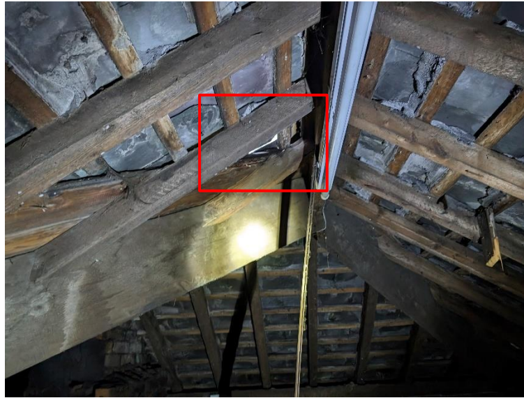
PLATE 5 SHOWING SLIPPED TILE
