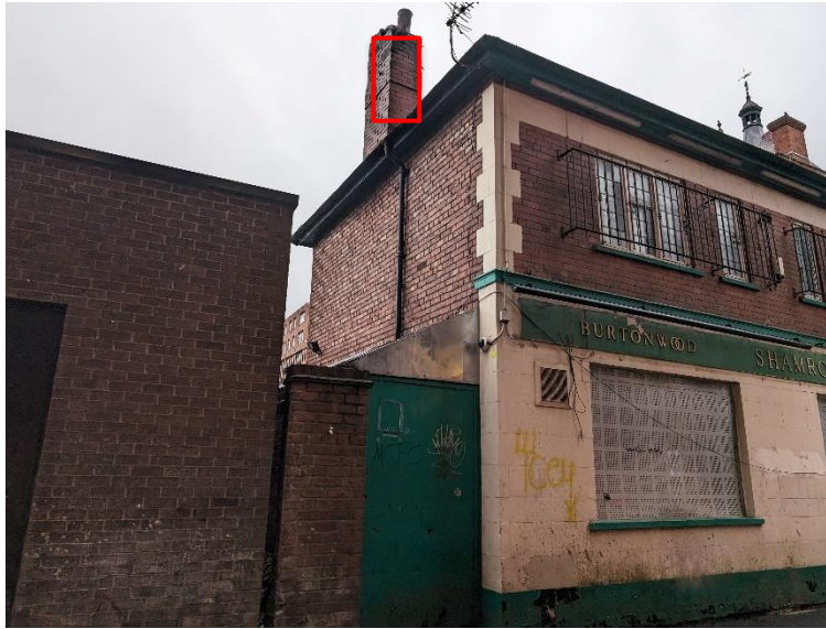
PLATE 10 SHOWING DAMAGED BRICKWORK ON CHIMNEY BREAST
