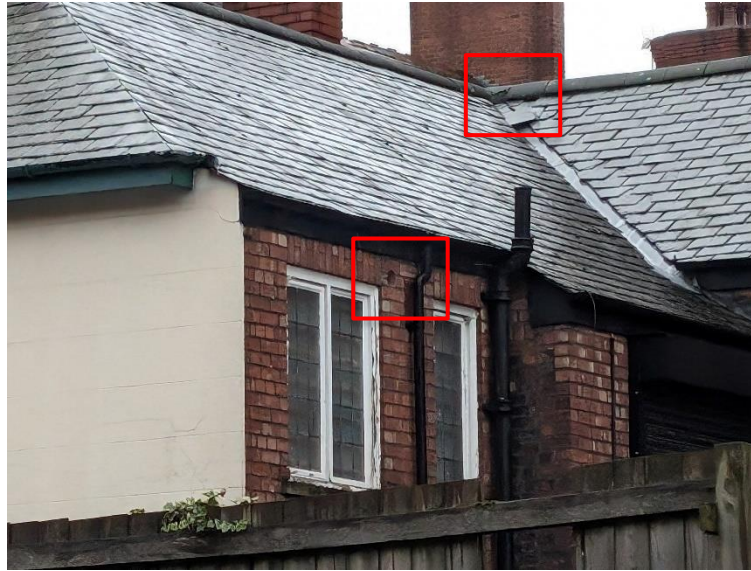
PLATE 7 SHOWING HOLE INTO WALL ON EASTERN ASPECT
