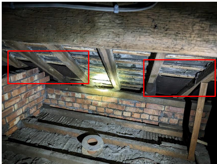
PLATE 4 SHOWING AREA OF LIFTED FELT
