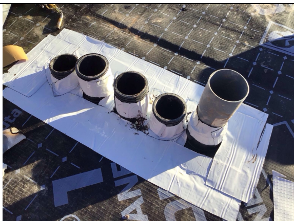
Detailed pipe penetrations
