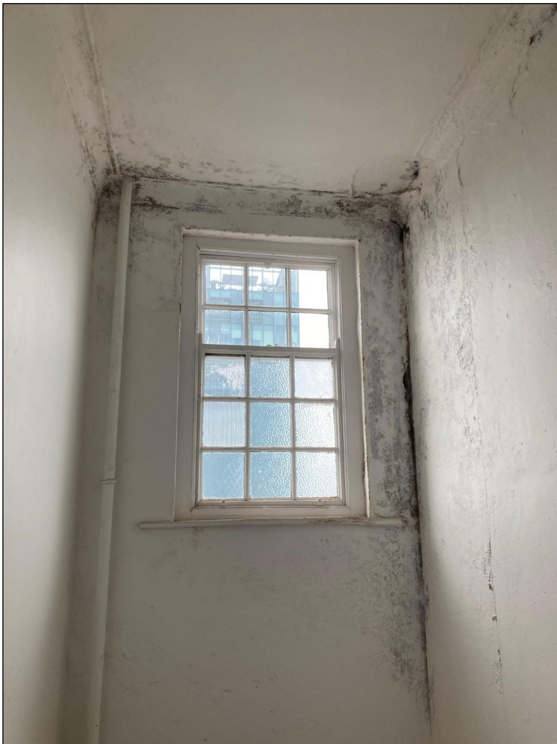
Deteriorating walls within caretaker's flat
