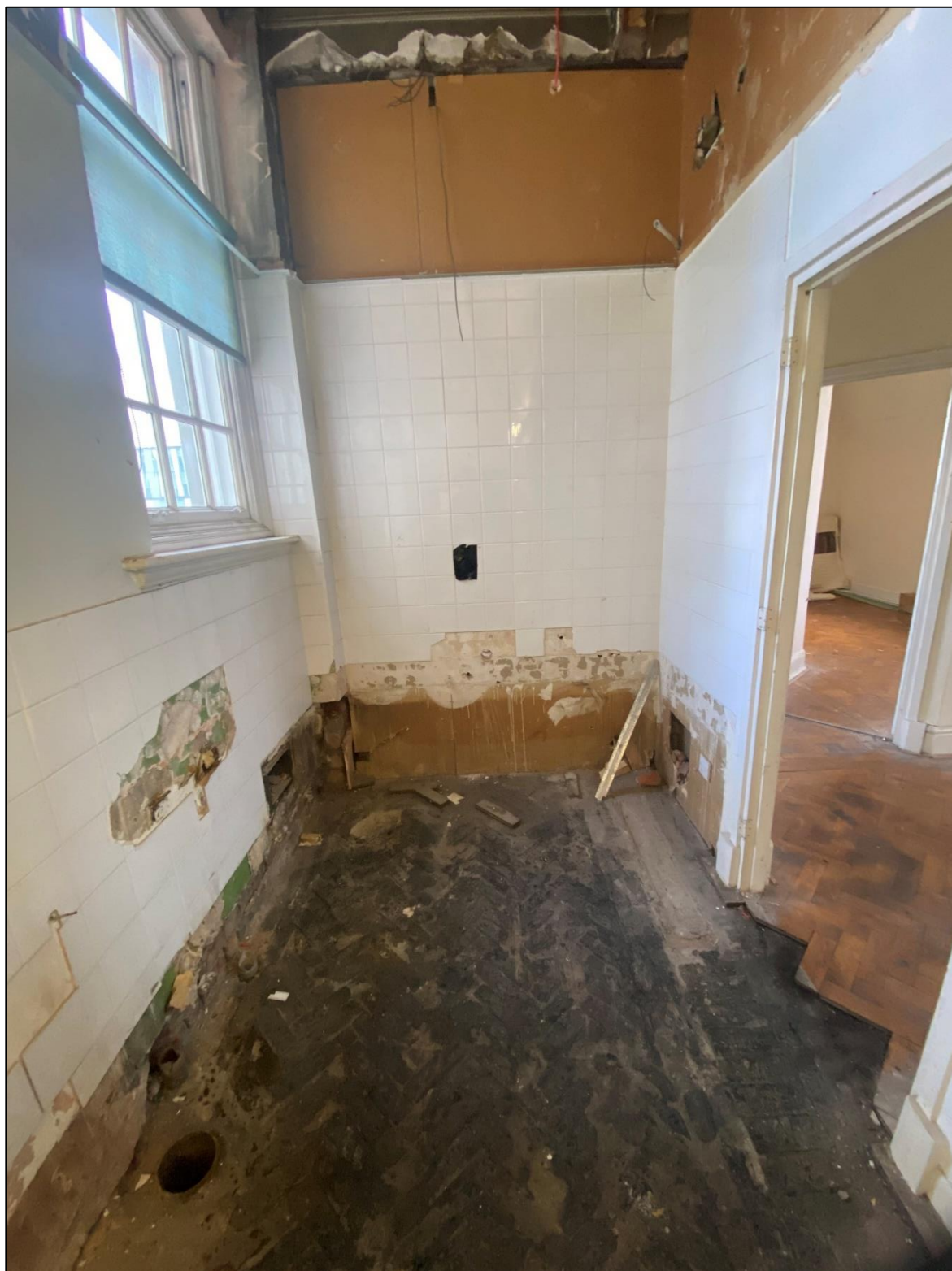
Caretaker's flat with deteriorating material
