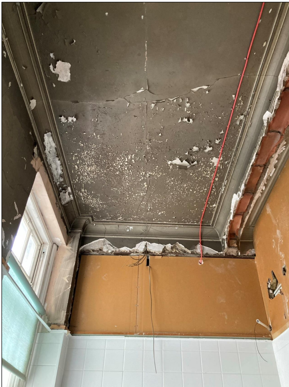
Deteriorating ceiling within caretaker's flat
