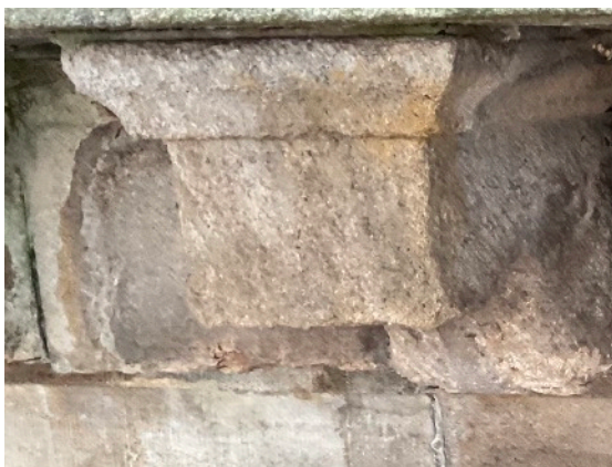
Most pointing to stonework has eroded. Where visible pointing is buff.
