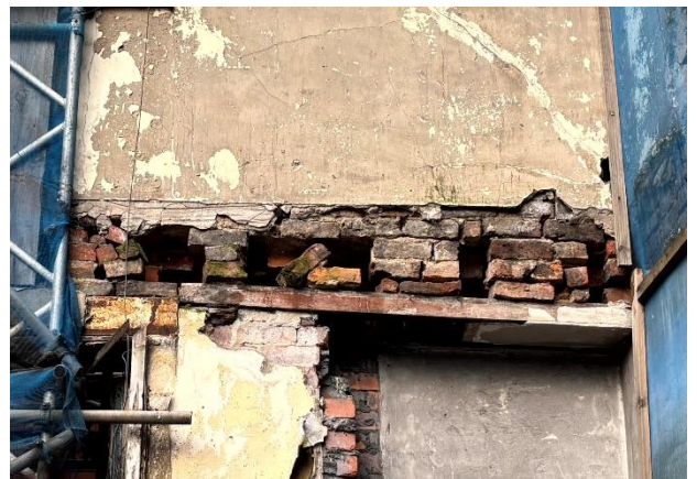
Damaged brickwork around first floor joist pockets (January 2025)
