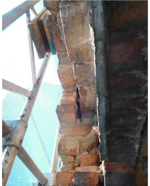
Unsupported brickwork of inner leaf above former window opening (April 2023)
