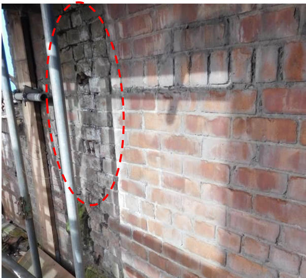
Very poor condition brickwork from missing rainwater pipe (April 2023)
