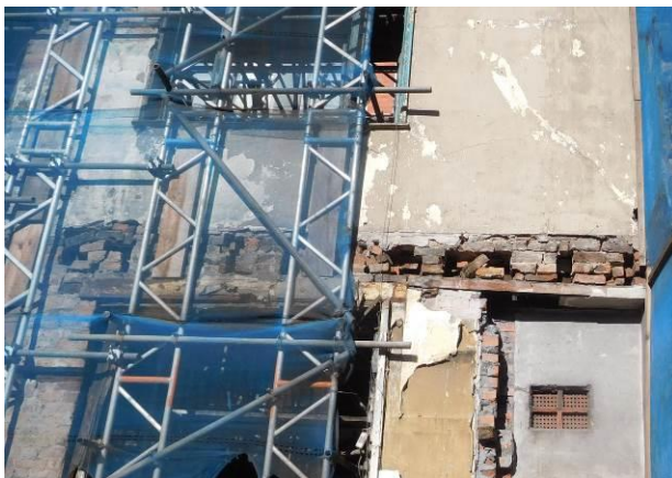
Damaged brickwork around first floor joist pockets (April 2023)
