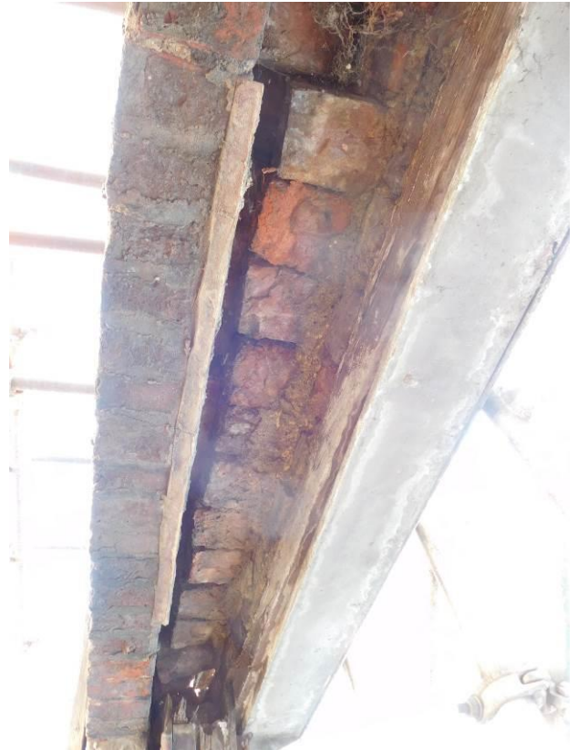
Unsupported window head separating from outer leaf of brickwork (April 2023)
