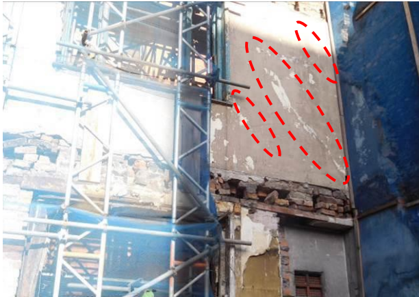
Cracking in panel above side entrance doorway (April 2023)
