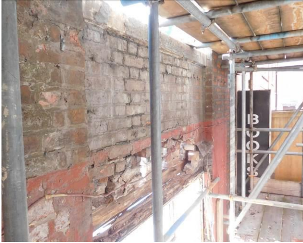
Distressed brickwork above rotten lintel (April 2023)
