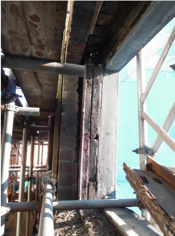
Rotting timber frame leaving unsupported brickwork (April 2023)
