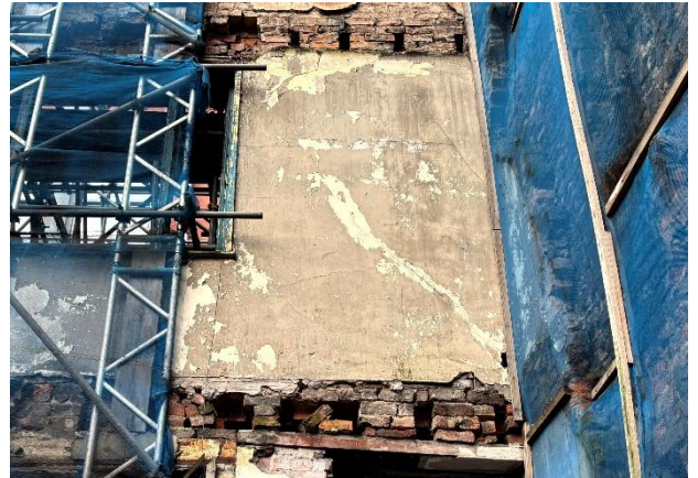
Cracking in panel above side entrance doorway (January 2025)
