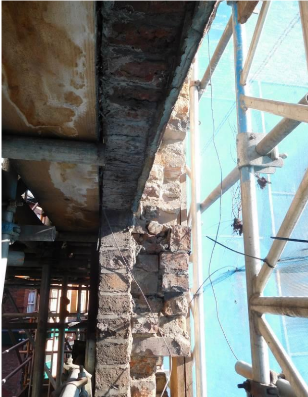
Damaged brickwork reveal (April 2023)
