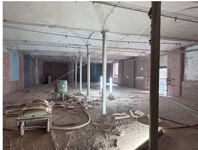
Figure 56. First-floor, Bradford Road. Sample 14 was modern paint.
