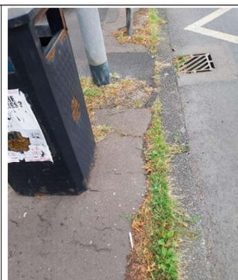
Photo 23 – Cracking to pedestrian surface course. Shallow vegetation to kerb edging.
