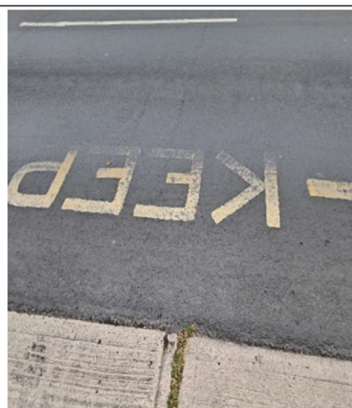
Photo 25 – Faded road markings to highway. Shallow vegetation between concrete surface course
