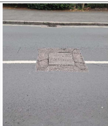
Photo 27 – Cracking to surround of highway inspection chamber. Cover and surface raised
