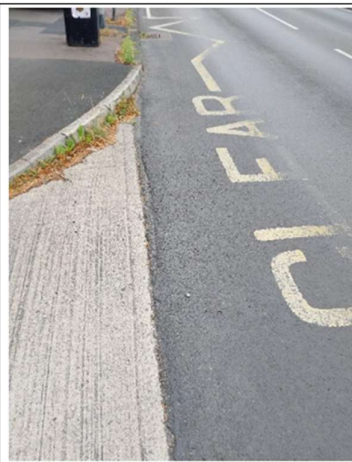
Photo 19 – Minor unevenness to abutment of tarmac surface course. Faded road markings.
