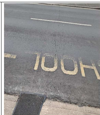
Photo 24 – Minor surface course cracks along highway surface course.
