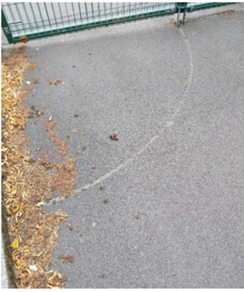
Photo 5: Impact damage from opening and closing of main gate.
