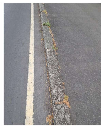
Photo 17 – Generally uneven concrete kerb edgings. Road markings in fair condition.
