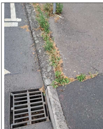
Photo 13: Minor cracking to pedestrian footpath. Road markings visible.
