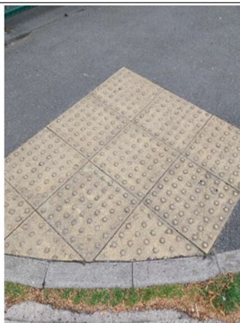
Photo 20 – Aged tactile paving. Shallow vegetation with exposed concrete dropped kerb.
