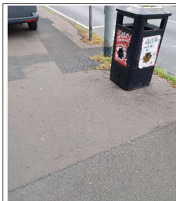
Photo 22 – Cracking to pedestrian surface course.
