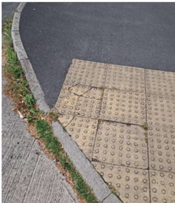
Photo 10: Cracking noted to tactile paving. Shallow vegetation to concrete kerb edging.
