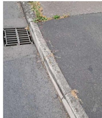
Photo 12: Evidence of newer laid tarmac and edging.
