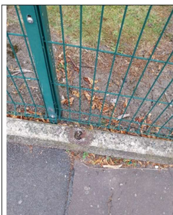
Photo 16 – Impact damage to concrete kerb edging from previous fence installation.
