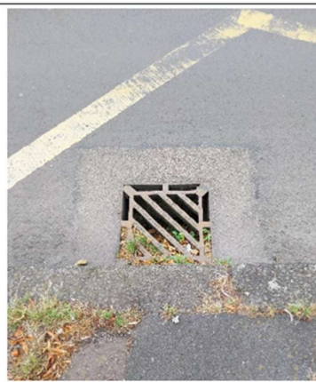
Photo 29 - Shallow vegetation noted to gully and kerb edging. Faded road markings.
