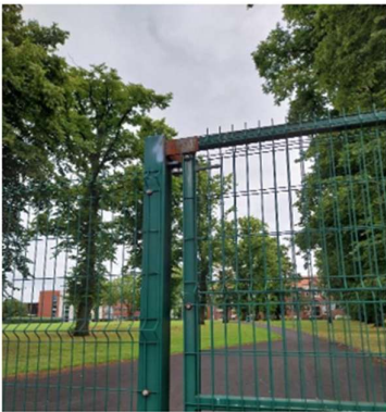
Photo 8: Corrosion evident to main entrance gate hinge.
