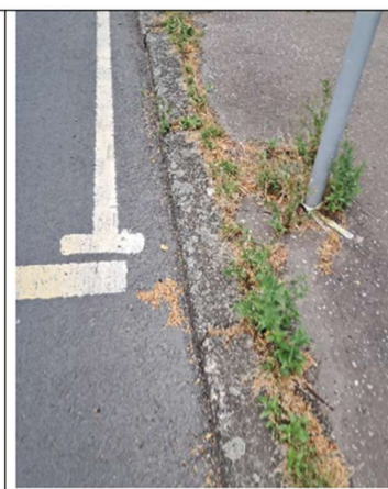
Photo 14: Aged condition of kerb edgings, generally uneven with shallow vegetation.
