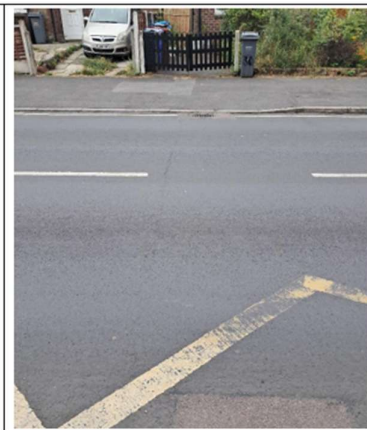
Photo 30 - Minor surface course abrasions to highway. Faded road markings.
