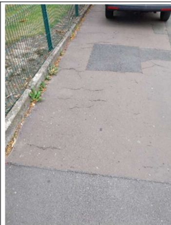
Photo 21 – Cracking to tarmac pedestrian surface course.
