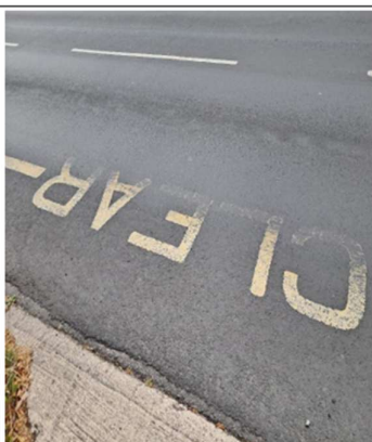
Photo 26 – Faded road markings to highway.
