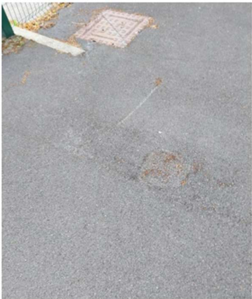
Photo 6: 3-4mm shallow surface damage.
