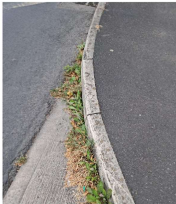
Photo 11: Minor cracking to abutment of tarmac and concrete surfaces.
