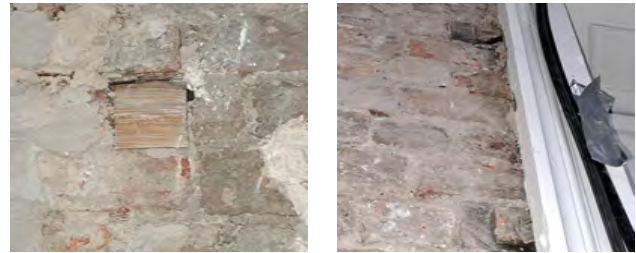
Figure 2 Timber embedded in the brickwork
