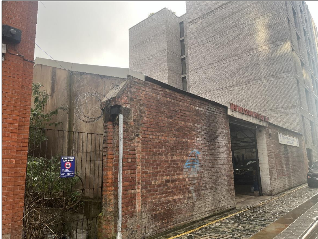
Plate 3 – Front elevation of site, with minor damage noted to external side (north-west) walls.
