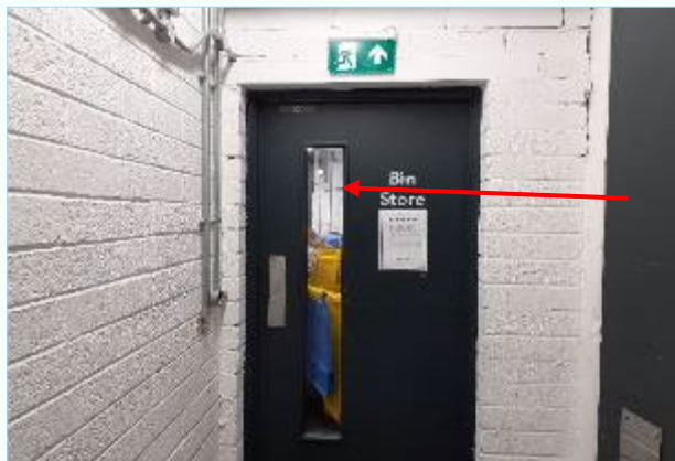
Lower Ground bin store door where FDP1 is located.
