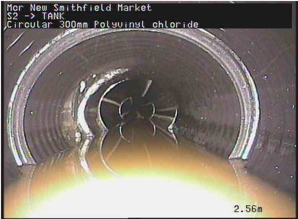
S2X_a6d13c1d-3f1f-4086-8546-778b02011d1c_20241104_092 512_015.jpg, 00:00:20, 2.56 m Open joint, medium
