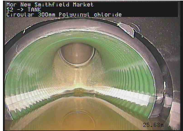
S2X_f7222f66-3294-4dcc-8600-5484e84aa56d_20241104_092 943_480.jpg, 00:04:14, 25.68 m Open joint, medium
