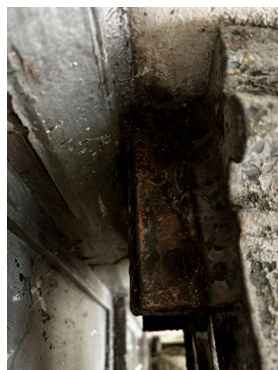
Figure 3 - Evidence of corrosion & detritus on the connection detail
