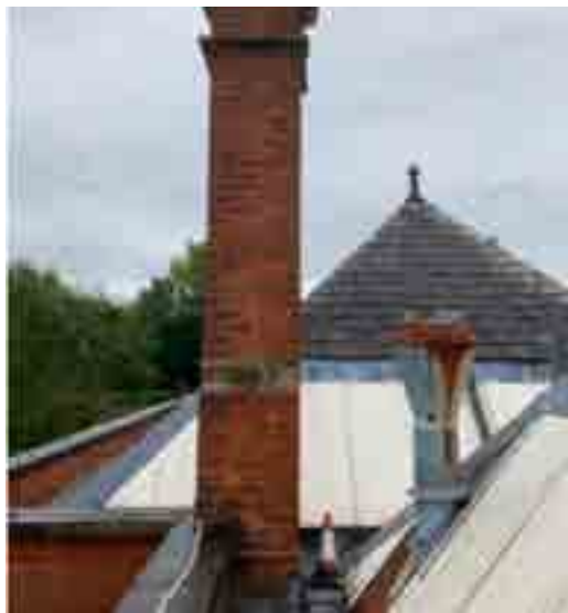
Image 1. Illustration of the close proximity of the roof parapet to the rooflight within the pitched roof.
