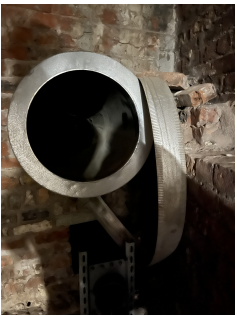
Image B - redundant duct to be removed and brickwork reinstated.
