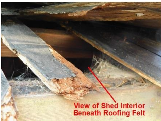
PHOTO 29 Underside of Part of Shed Roof
