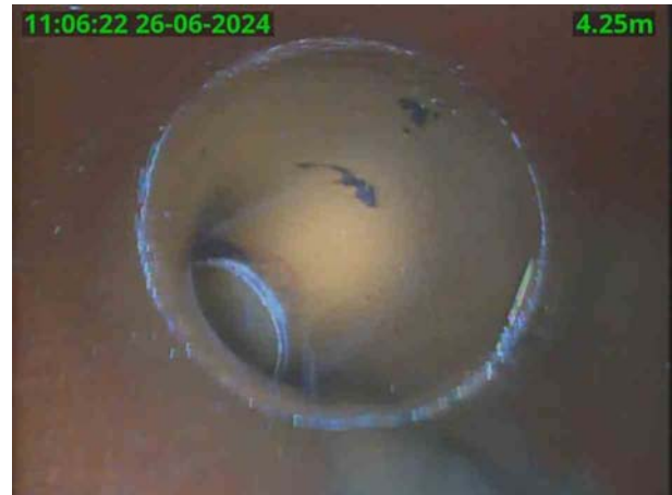
MH F1X_a8ce3e10-c9cc-40ed-a451-680f2b5ee1b9_20240626_15 0229_752.jpg, 00:01:21, 4.25 m Line deviates left
