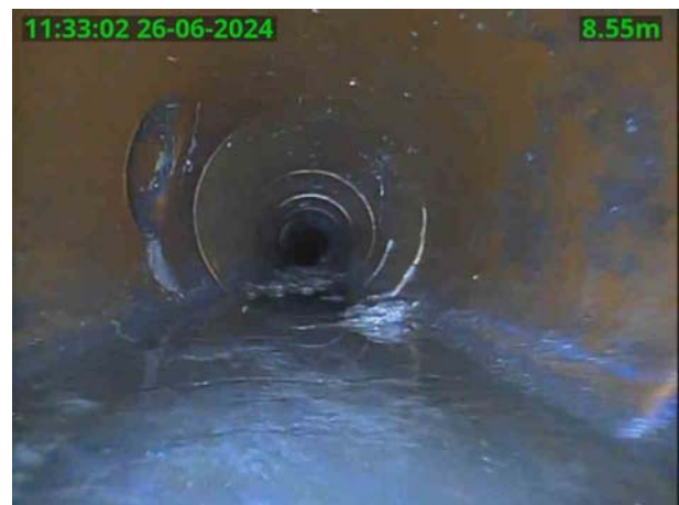
MH 8301X_e796bcff-1260-436c-b779-d81b2cfa5fdb_20240626_14 4302_287.jpg, 00:00:49, 8.55 m Junction at 9 o'clock, 150mm dia
