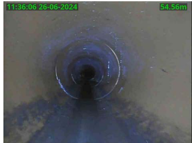
MH 8301X_34cd5b4f-5b8b-4c72-8450-9d3462c29043_20240626_145415_879.jpg, 00:03:53, 54.56 m Settled deposits, fine, 10% cross-sectional area loss, finish
