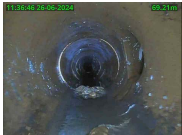
MH 8301X_14b84926-f9e4-4074-9350-39fd3f18fa27_20240626_145624_617.jpg, 00:04:33, 69.21 m Junction at 3 o'clock, 150mm dia
