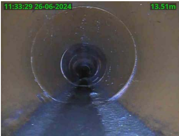
MH 8301X_d7274702-4543-4502-8448-ebef90335ff_20240626_1 44349_534.jpg, 00:01:16, 13.51 m Settled deposits, fine, 10% cross-sectional area loss, finish
