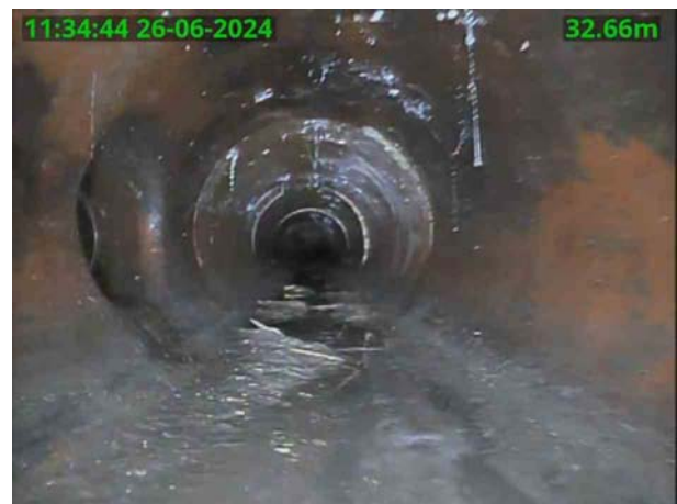
MH 8301X_cbe1a71a-553f-446a-a8bf-4aec8d82de09_20240626_1 44906_702.jpg, 00:02:31, 32.66 m Junction at 9 o'clock, 150mm dia
