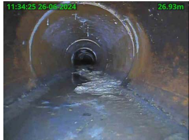
MH 8301X_57444b3b-2df2-4a46-a43f-daa3cc96a4d9_20240626_1 44747_748.jpg, 00:02:12, 26.93 m Settled deposits, fine, 10% cross-sectional area loss, start
