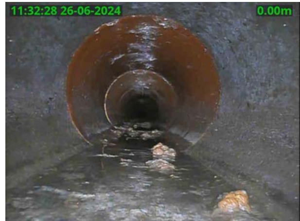
MH 8301X_0366b74d-69e5-4719-b16e-dea494ff9b71_20240626_1 44101_190.jpg, 00:00:15, 0.00 m Settled deposits, fine, 10% cross-sectional area loss, start
