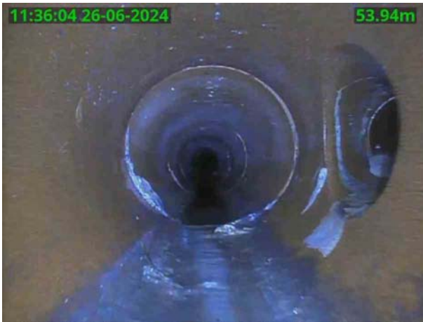
MH 8301X_1d406252-4052-49da-b57a-9a0b02d84696_20240626_145352_648.jpg, 00:03:51, 53.94 m Junction at 3 o'clock, 150mm dia
