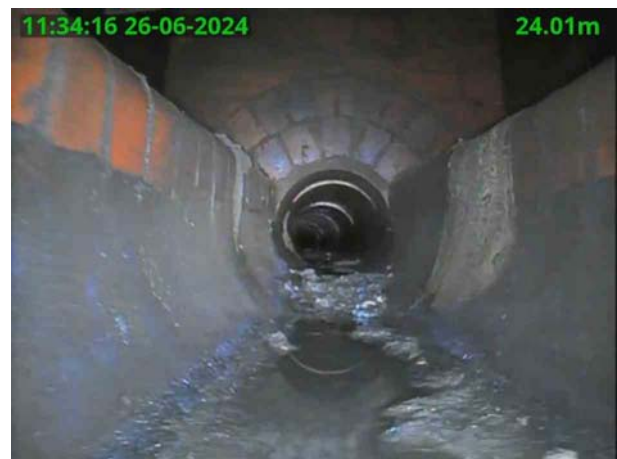
MH 8301X_e2bffc1c-c488-4d4a-a761-1ca0d67be1db_20240626_1 44622_777.jpg, 00:02:03, 24.01 m General remark, MH NO REF ON DRAWING
