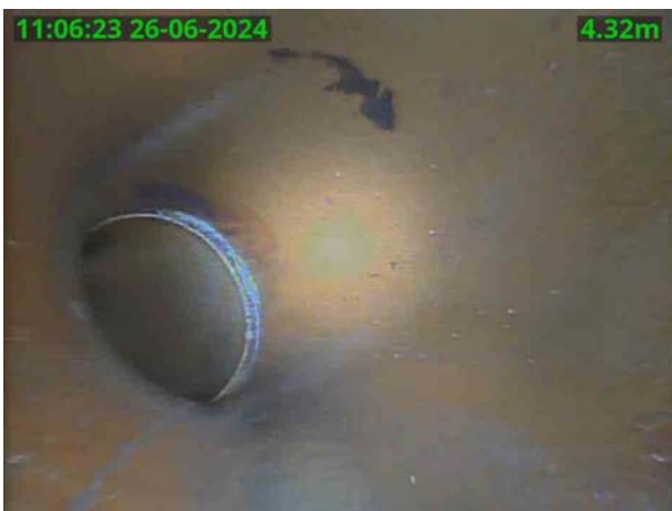
MH F1X_2b94b9bf-0f11-4e16-8521-3a30e24cab4a_20240626_15 0252_061.jpg, 00:01:22, 4.32 m Line deviates down
