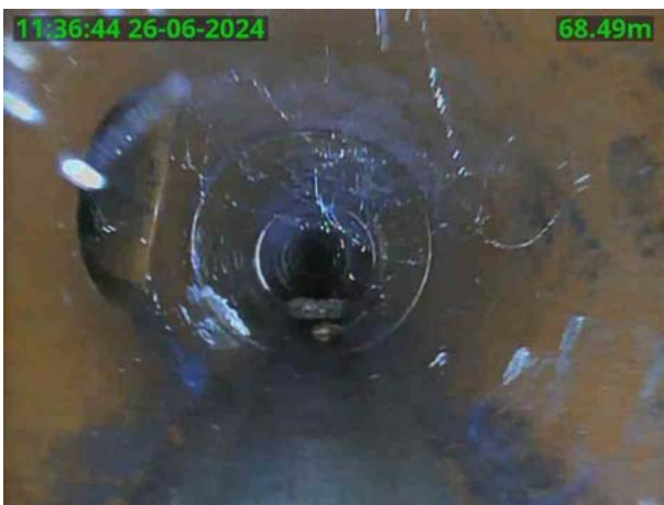
MH 8301X_fb132325-d32f-4a74-a2f1-678e4e2ca0ab_20240626_145525_565.jpg, 00:04:31, 68.49 m Junction at 9 o'clock, 150mm dia
