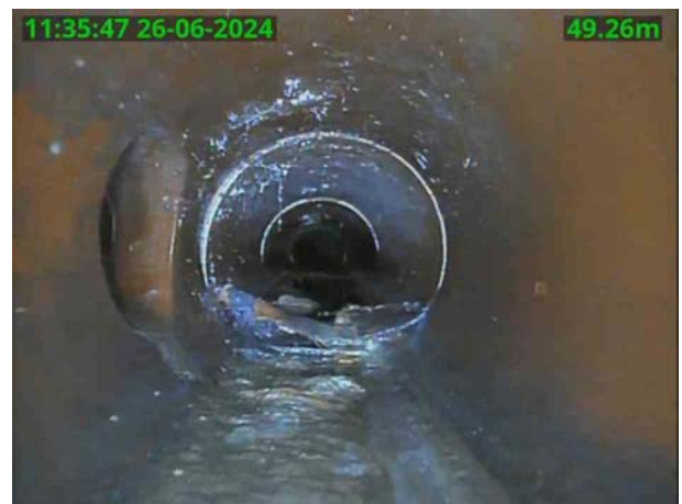
MH 8301X_57bca2c4-0a31-49cc-b1bd-21747c1f46ba_20240626_1 145236_788.jpg, 00:03:34, 49.26 m Junction at 9 o'clock, 150mm dia
