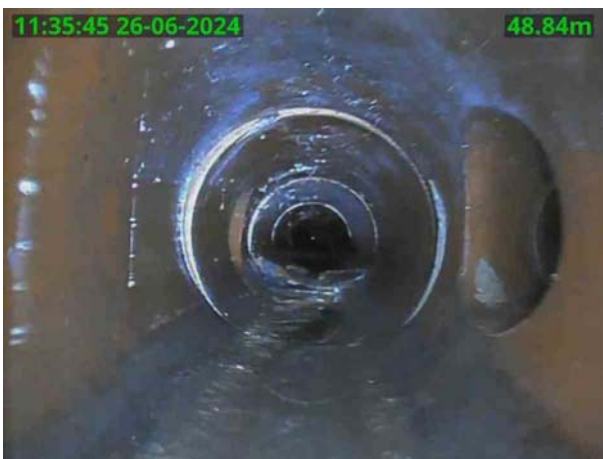
MH 8301X_00de4aff-2cc9-42d3-b5c9-598e5489bd0c_20240626_1 45200_154.jpg, 00:03:32, 48.84 m Junction at 3 o'clock, 150mm dia
