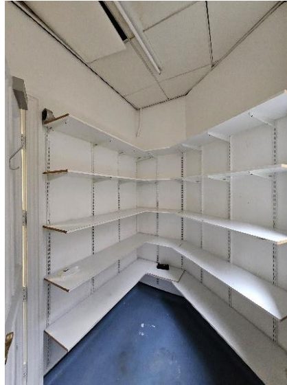
Figure 23: Store Room G.002
