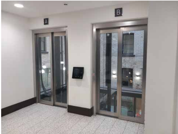
3.51 floor, Hanover Building - lifts
