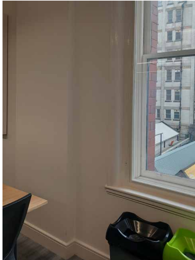
3.48 1 st floor, E Block - pilaster vent system
