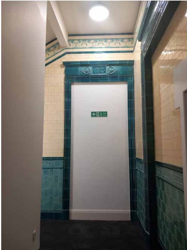
3.33 Hanover Building, Bloom Street staircore - blocked openings
