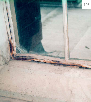
Image 106 Steel window showing severe corrosion to the bottom rail of the frame and distortion from 'rust jacking' which has cracked the glass.
