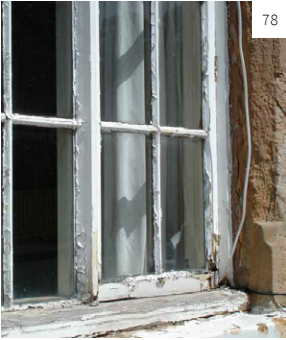
Images 76-78 76. Some of the problems to look out for when inspecting older windows. 77. A double hung sash window lacking maintenance but still easily capable of being overhauled. 78. Lack of maintenance has resulted in lost putties to glazing and rot at the base of the window frames all capable of repair. Cables fed through the base of the frame have allowed water to enter and contribute to the rot.
