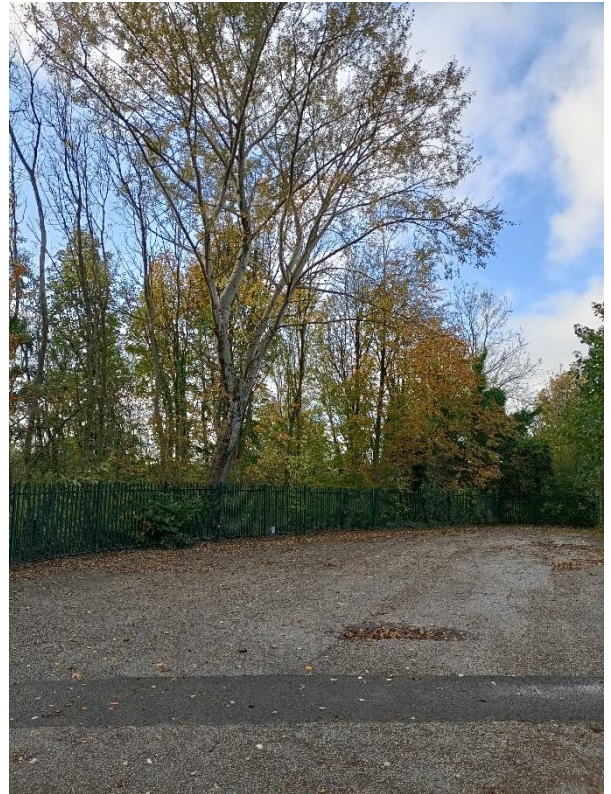
Figure 2.4: Linear patching of the tarmac car park surface indicating buried utilities.
